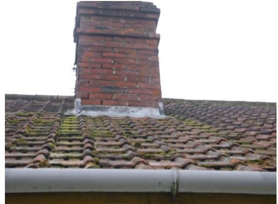
Photograph 4. Gaps under lead flashing around chimneys.
