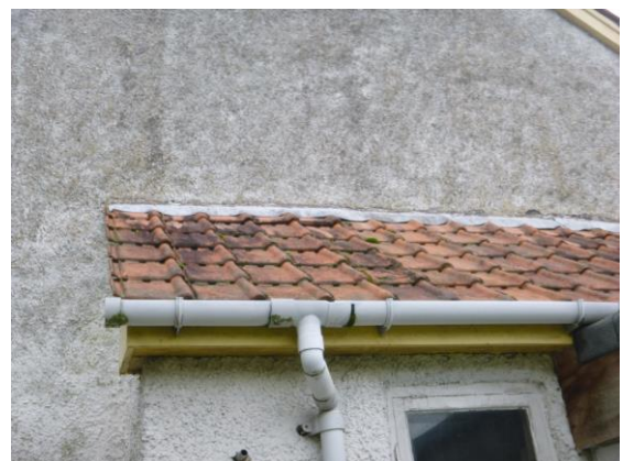
Photograph 8. Lifted pantiles on rear porch roof.
