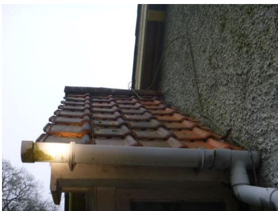
Photograph 7. Lifted pantiles on bay window roof.
