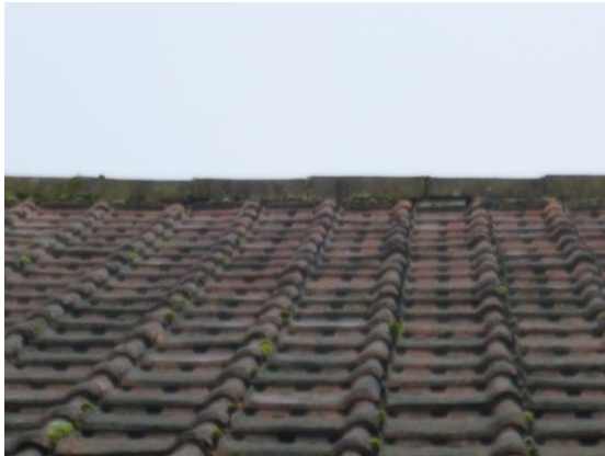
Photograph 3. Several small gaps under roof and ridge tiles.
