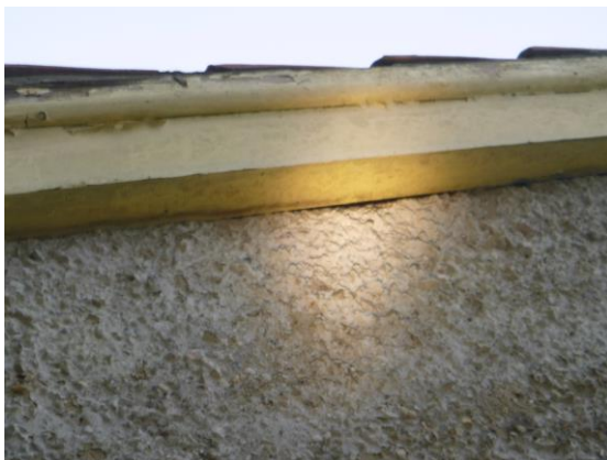
Photograph 5. Gap behind fascia on rear gable end.
