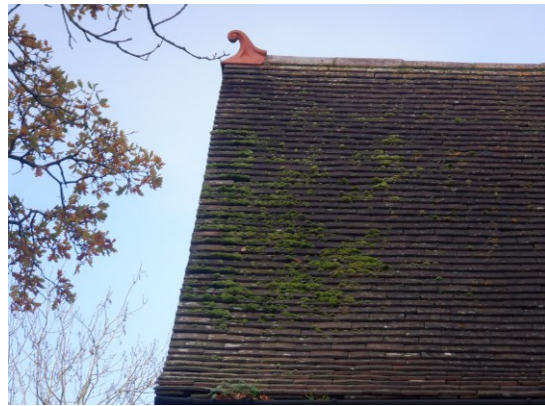
4. Uneven row of clay roof tiles along the southwest verge, viewed from the southeast.
