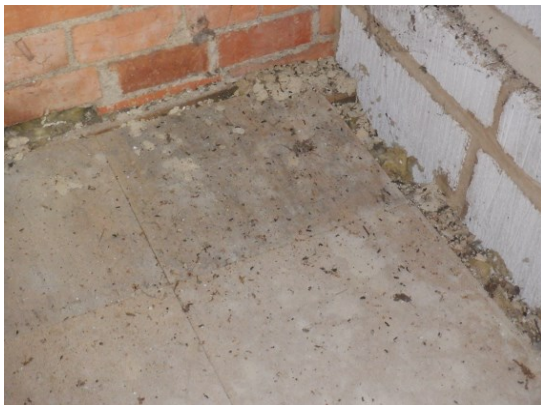
27. Approximately 200 - 300 medium-sized bat droppings at the base of the northeast party wall.
