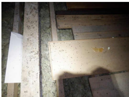
24. Medium-sized bat droppings scattered throughout the roof void.
