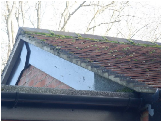
5. Frequently lifted clay roof tiles on the existing rear extension, viewed from the west.
