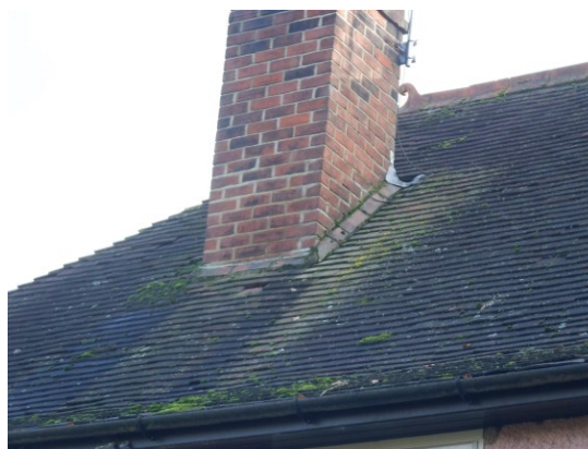
10. Gap between clay roof tiles and lead flashing to the rear of the chimney, viewed from the west.
