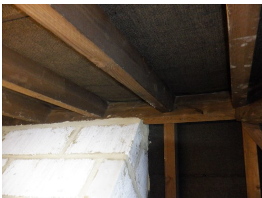
19. Slight gaps between bitumen felt and ridge which are both connected to an internal blockwork wall.
