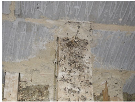
26. Approximately 300 - 400 medium-sized bat droppings at the base of the southwest gable wall.
