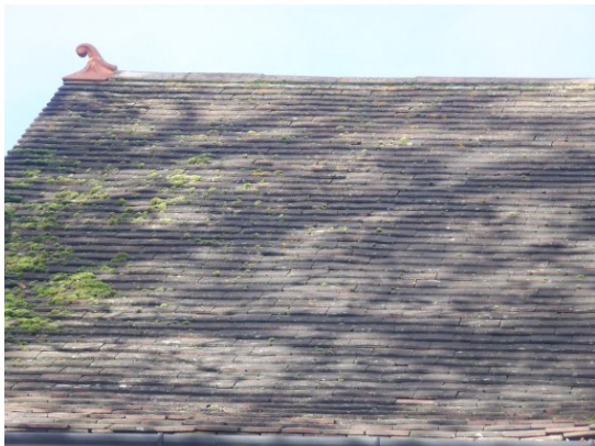
3. Frequently lifted, damaged or missing clay roof tiles, viewed from the southeast.
