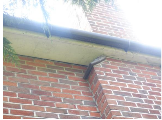
Photograph 7. Gap between soffit and brickwork (eastern elevation).
