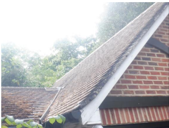
Photograph 10. Soffit tight to brickwork gable of garage (eastern elevation).
