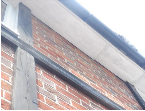
Photograph 6. Gap between soffit and brickwork (rear elevation).
