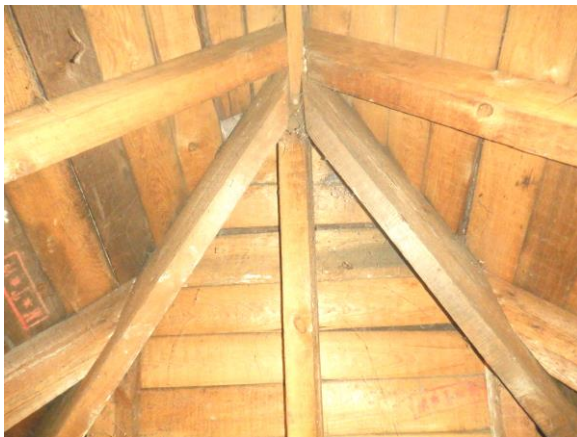
Photograph 13. Lightly cobwebbed timber sarking at the eastern end (first roof void).
