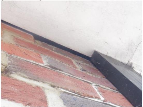
Photograph 8. Small-sized bat dropping on brickwork below soffit (rear elevation).
