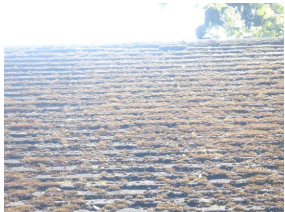
Photograph 5. Mossy clay roof tiles on garage (front elevation).
