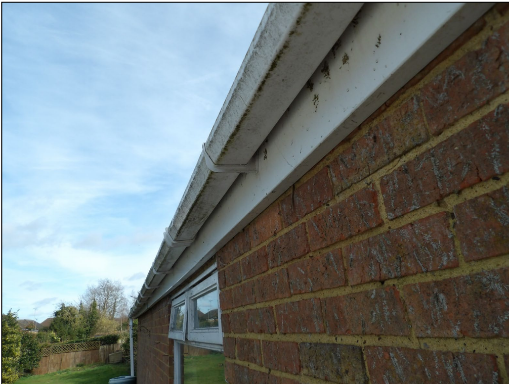
Figure 10. Example sealed fascias on garage. 3 Northbury Avenue, Ruscombe. 25.02.25
