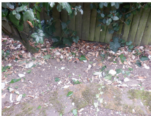
Photograph 7. Gaps at base of timber panel fencing.
