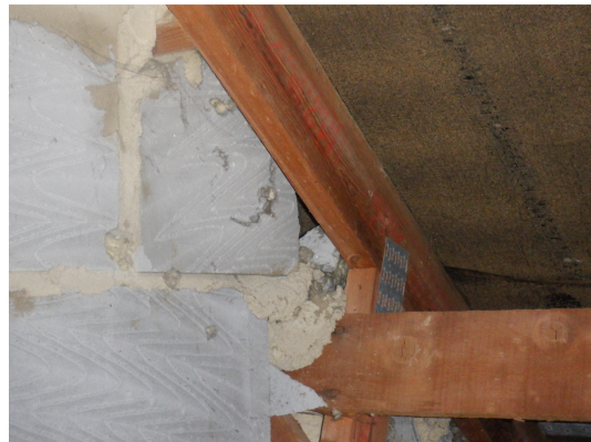
Photograph 16. Gaps around edges of the blockwork gables (roof void).
