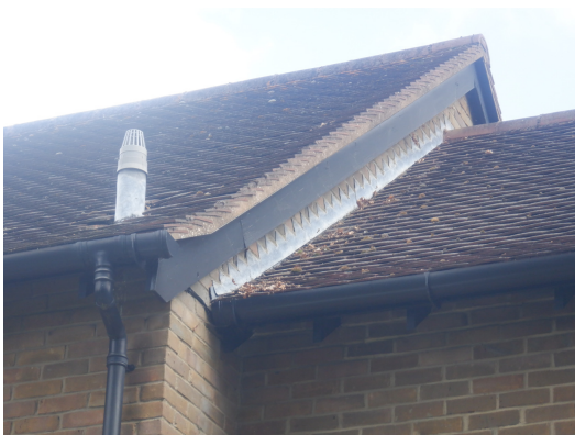
Photograph 3. Lifted clay roof tiles around flue pipe with fully intact ridge and verge mortar (rear elevation).
