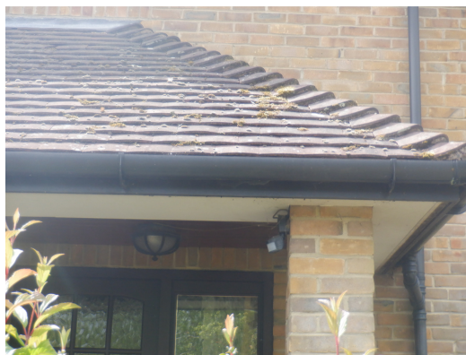
Photograph 4. Hip mortar fully intact (front elevation).
