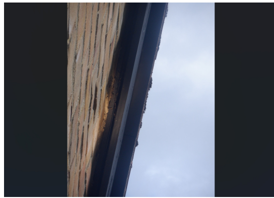
Photograph 8. Gaps behind timber fascia sealed with cement (northwest elevation).
