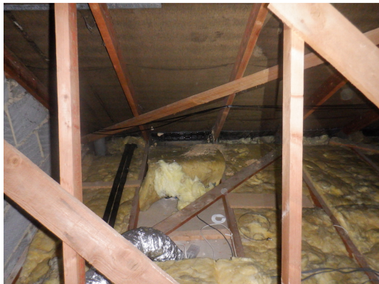
Photograph 15. Open eaves with daylight visible (roof void).
