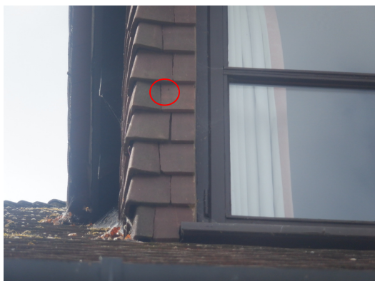
Photograph 10. Lifted corner hanging tiles with small-sized dropping on the dormer window above the garage (front elevation).
