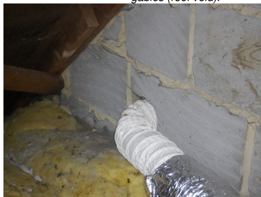
Photograph 17. Gaps around pipe in southeast blockwork gable (roof void).
