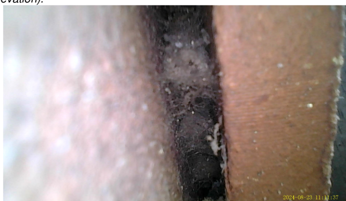
Photograph 12. Cobwebs behind lifted hanging tiles (front elevation).
