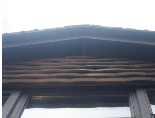
Photograph 11. Gaps under a few lifted tiles on the northwest dormer window (front elevation).
