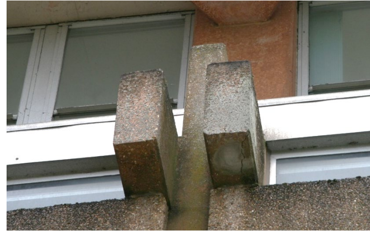
Example of Defect Type A2
