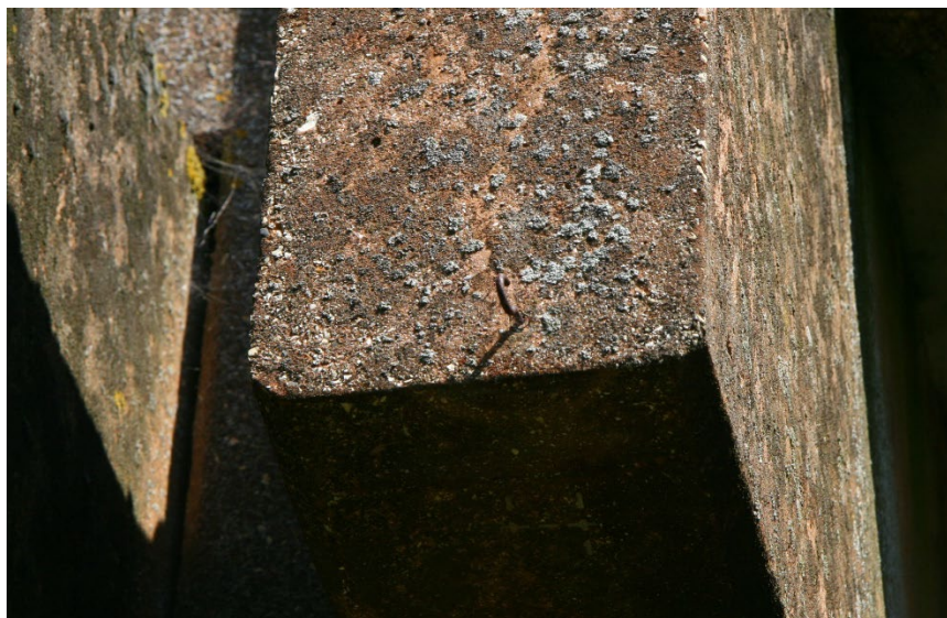
Example of Defect Type D2
