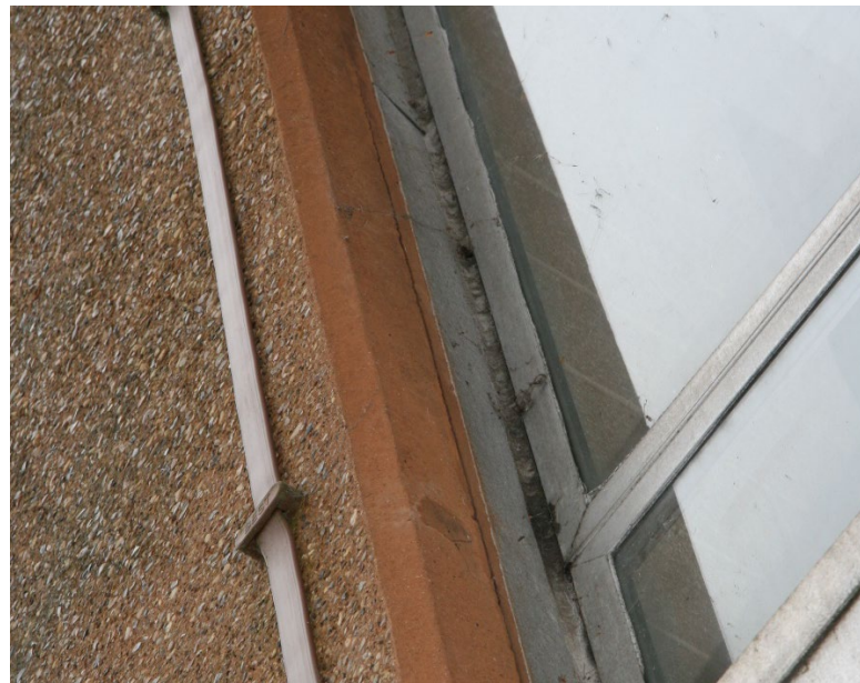
Example of Defect Type K1
