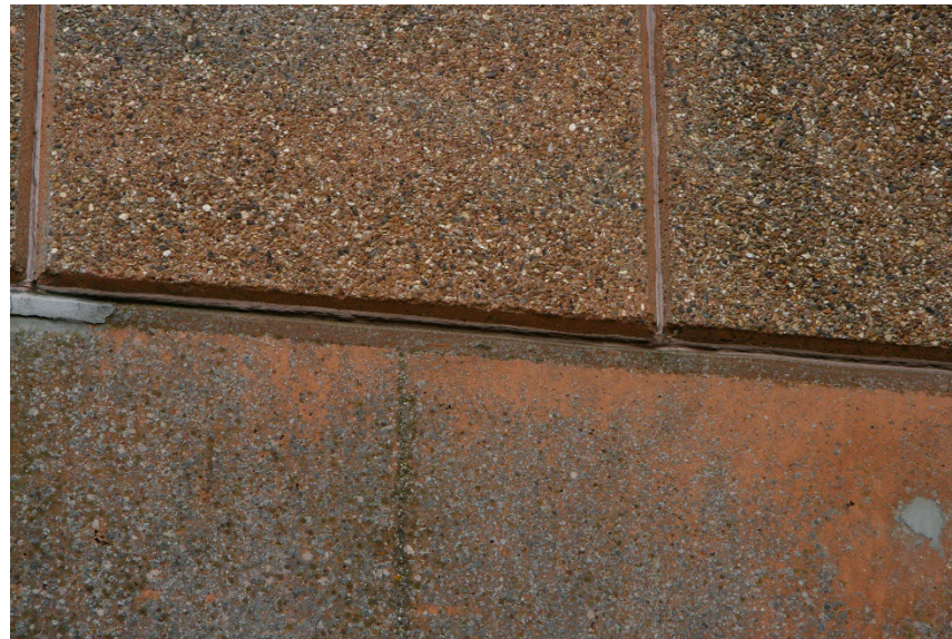
Example of Defect Type G1
