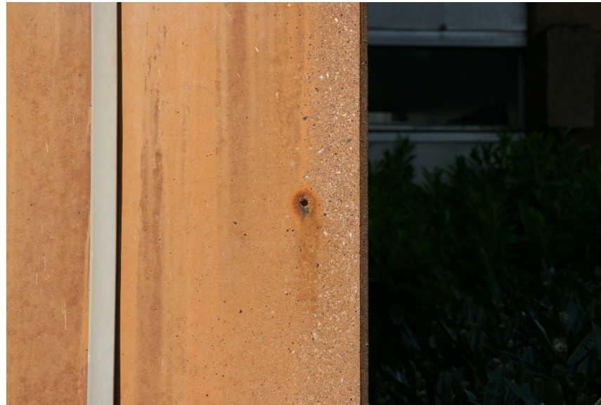
Example of Defect Type D1
