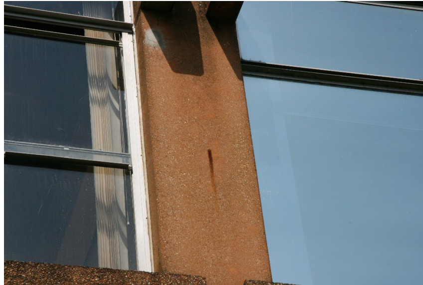
Example of Defect S2
