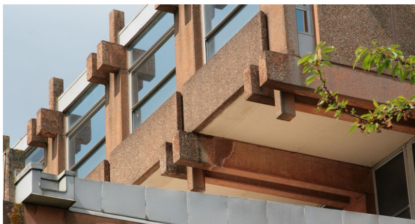
Example of Defect Type H2
