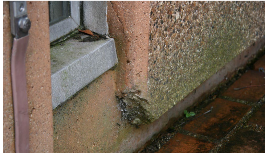
Example of Defect Type B3
