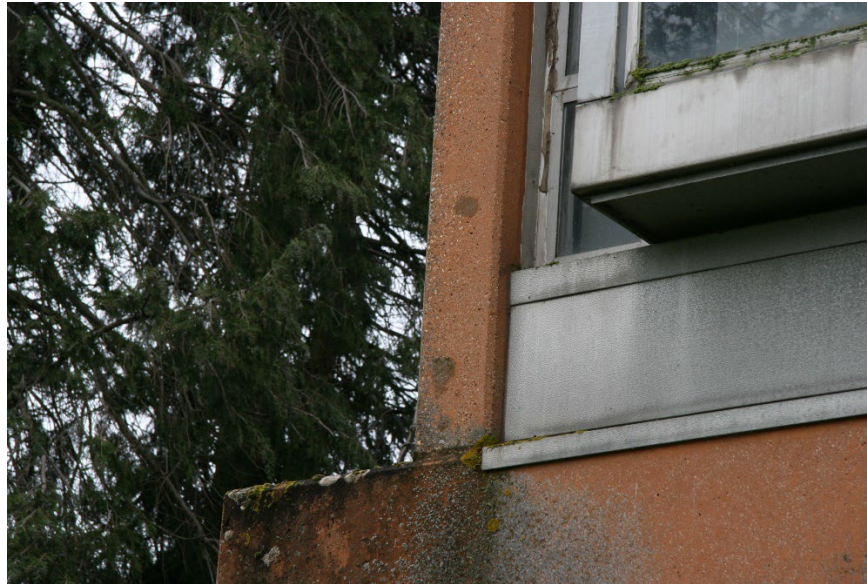
Example of Defect Type C2
