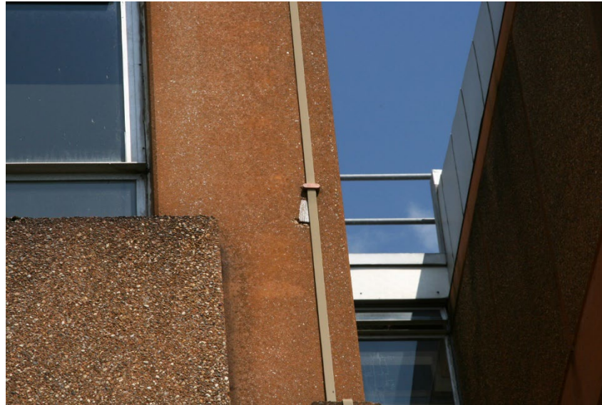
Example of Defect Type B5
