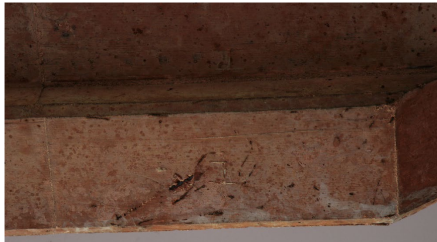
Example of Defect Type B6
