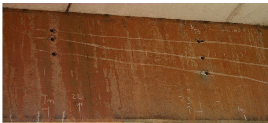
Example of Defect Type D3
