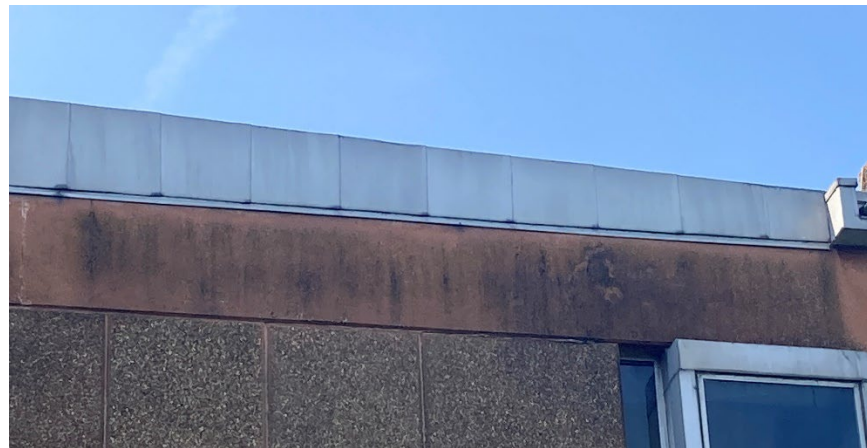
Example of Defect Type S1
