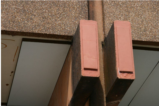
Example of Defect Type A1
