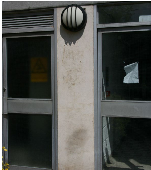
Example of Defect Type J1
