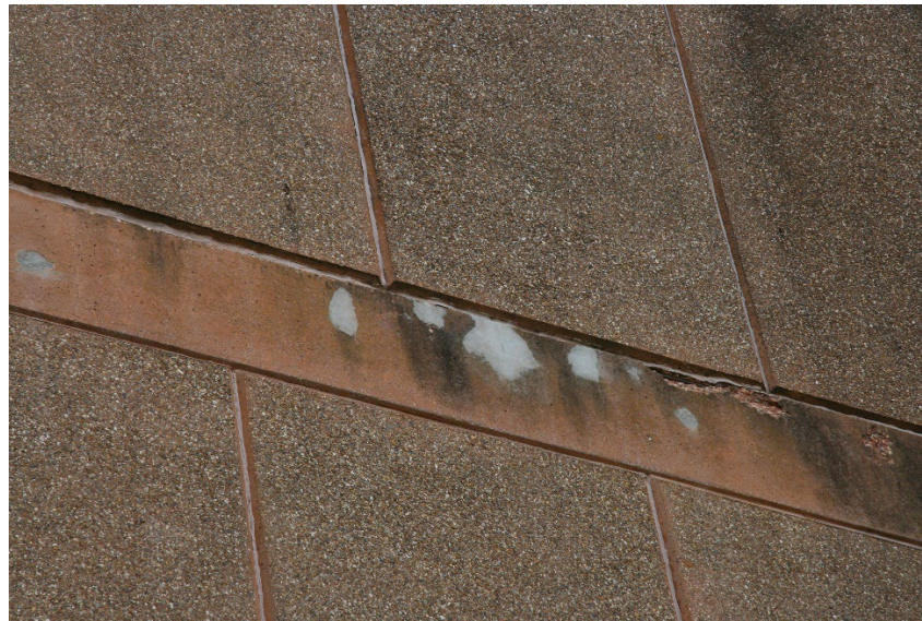
Example of Defect Type C1
