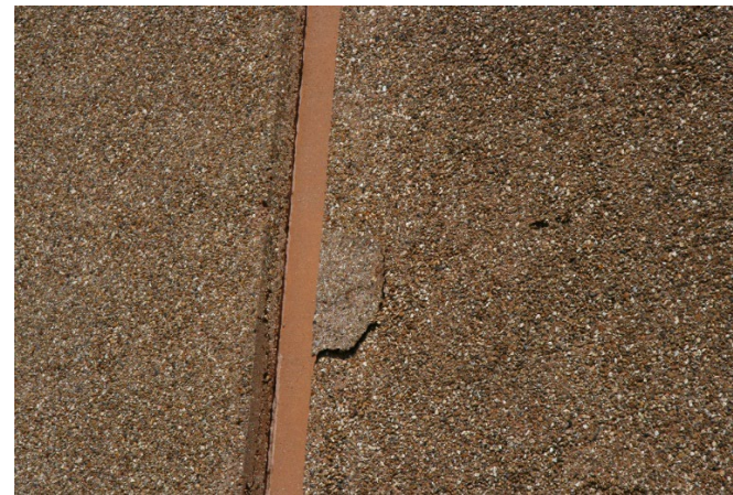
Example of Defect Type B2
