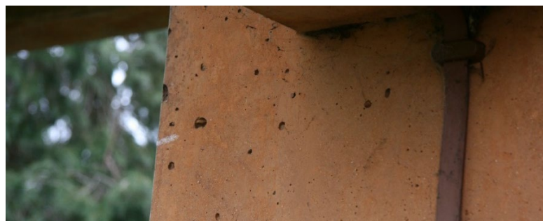
Example of Defect Type B4
