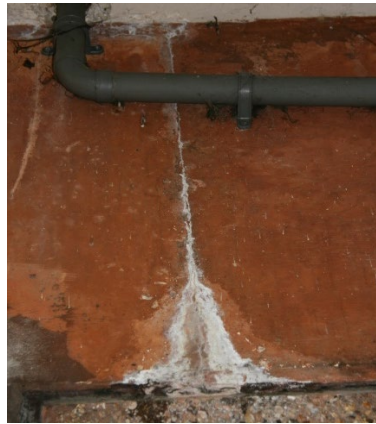
Example of Defect Type H1
