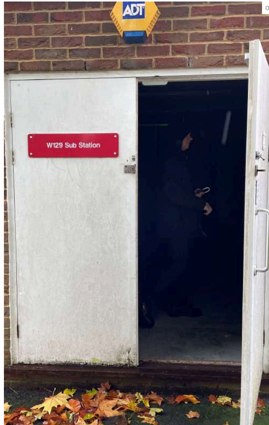
01 Photo of existing W129 Sub Station.
