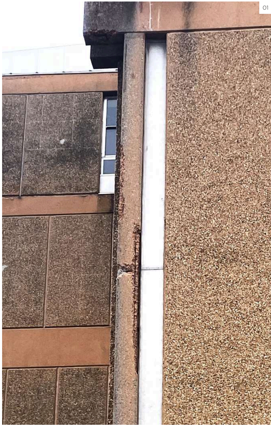
01 Concrete spalling and exposed reinforcement on external RC column.
