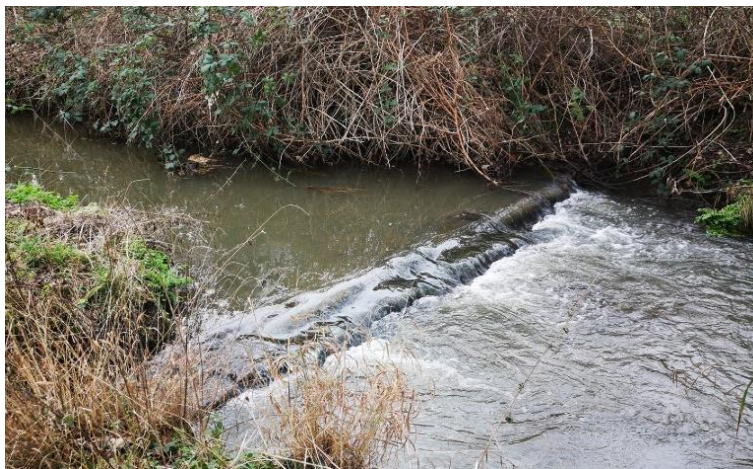
Figure 21 Weir formed from embedded foul sewer pipe.
