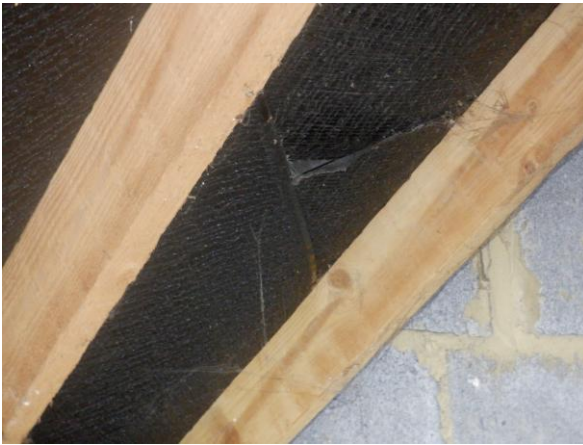
Photograph 11. Small tear in bituminous roofing felt (roof void).
