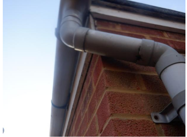
Photograph 8. Gap of limited extent under barge board on (eastern elevation).
