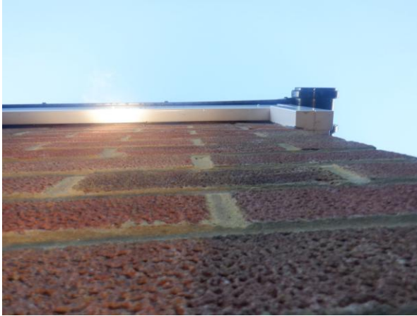
Photograph 7. Gap of limited extent under barge board on single storey rear extension (eastern elevation).
