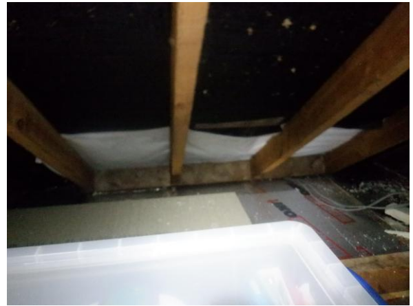
Photograph 12. Loosely overlapping breathable roofing felt where chimney was removed (roof void).
