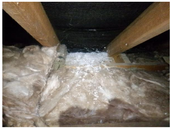
Photograph 10. Shredded insulation in eaves (roof void).
