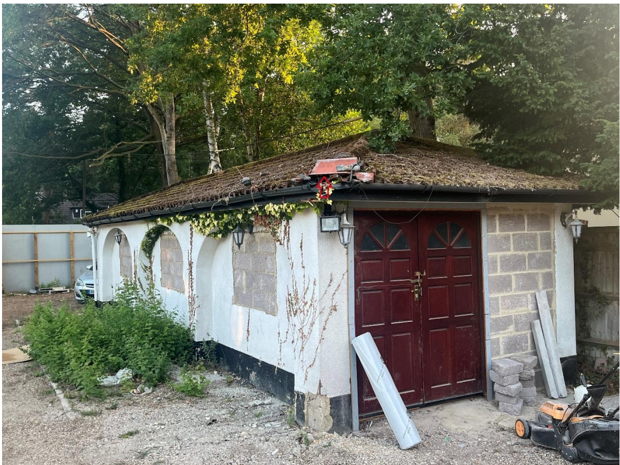
Figure 7. Garage looking southwest: Red arrow indicates potential openings for crevice roosting bats.
