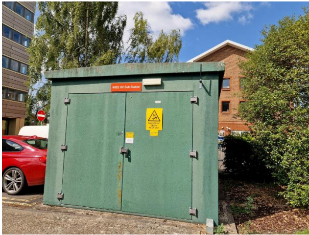
Figure 1. Front of Library Substation
