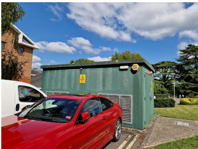
Figure 2. Side of Library Substation
