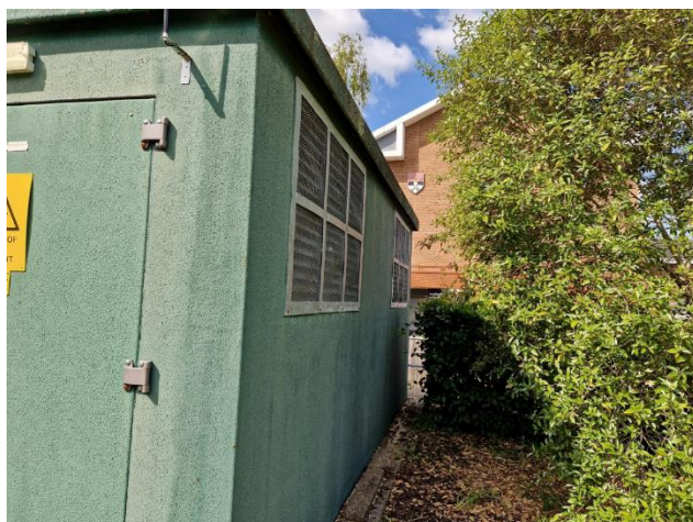
Figure 3. Side of Library Substation showing mesh covering
