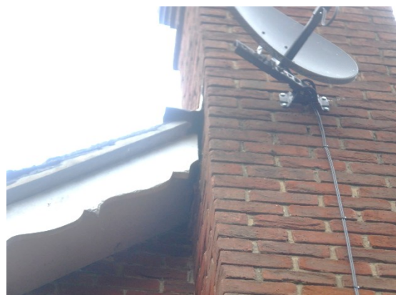
Photograph 13. Gap between soffit and brickwork chimney (south elevation).
