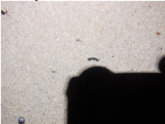
Photograph 22. Small-sized bat droppings at the base of the southern blockwork gable.
