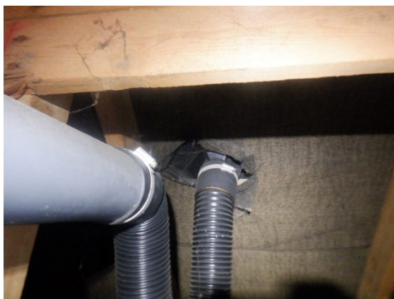
Photograph 17. Pipe sealed by a plastic guard.
