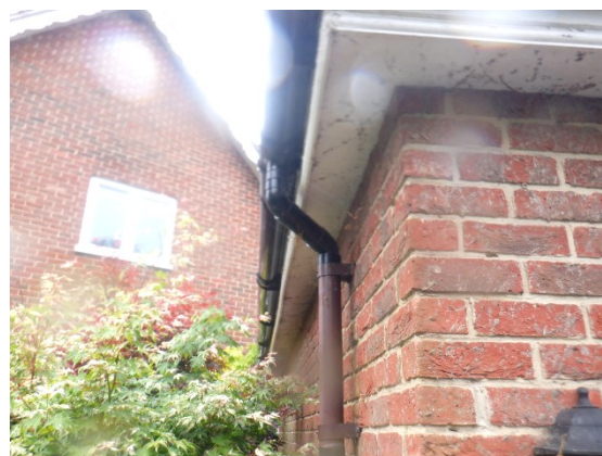
Photograph 15. Painted timber soffit sealed to brickwork around all sides of the garage.
