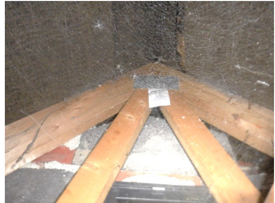
Photograph 21. Gaps at the apex and along the edges of the southern blockwork gable.
