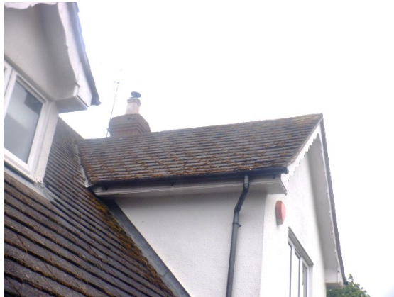
Photograph 3. Single lifted concrete tile (north elevation).
