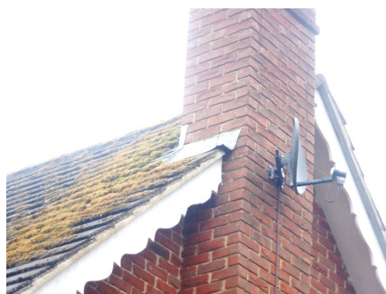
Photograph 9. Lead flashing lifted at the base of the chimney (front elevation).
