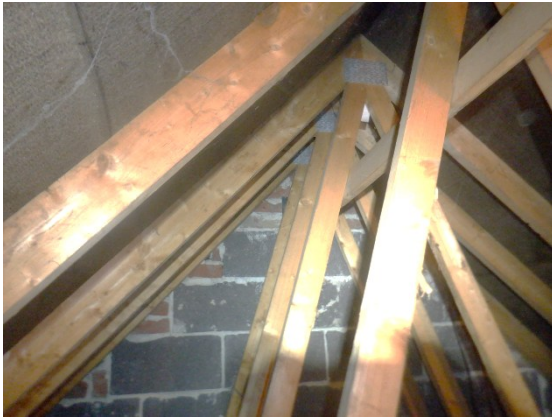
Photograph 20. Vent inaccessible at the northern blockwork gable.
