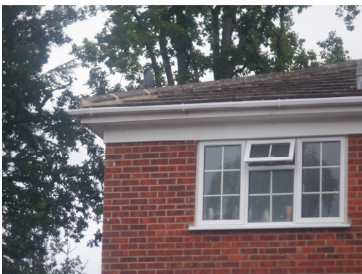
Photograph 5. Small area of repaired hip mortar (western elevation).
