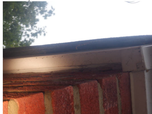
Photograph 12. Gap underneath the barge board on northern elevation with uPVC visible above (northern elevation).
