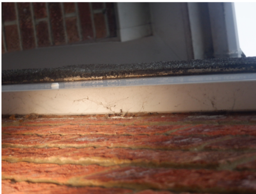
Photograph 11. Slight gap blocked with timber where the soffit box joined the wall on the northern elevation of the side extension.
