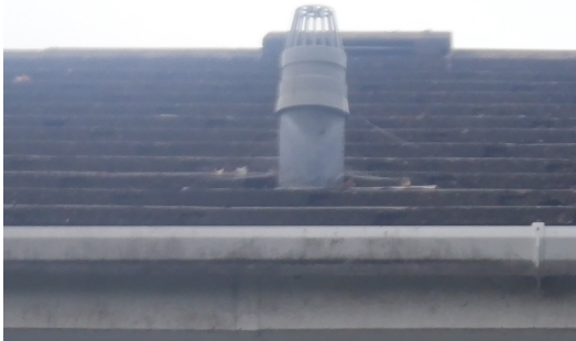
Photograph 9. Tight lead flashing on around the flute pipe (eastern elevation).
