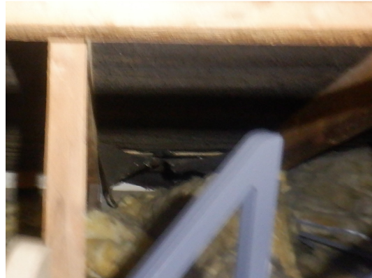
Photograph 15. Small area of loose fitting bitumen felt (roof void).
