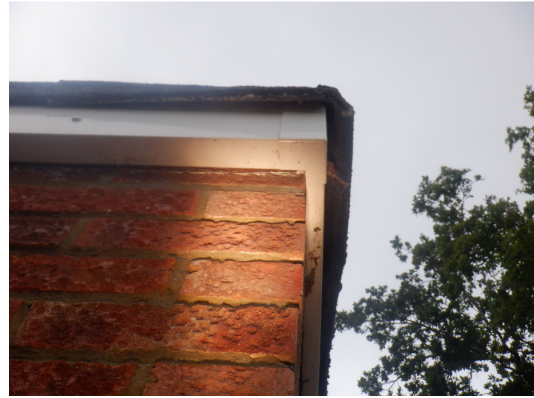
Photograph 10. Small superficial gap between bitumen roofing and uPVC bargeboard (eastern elevation).
