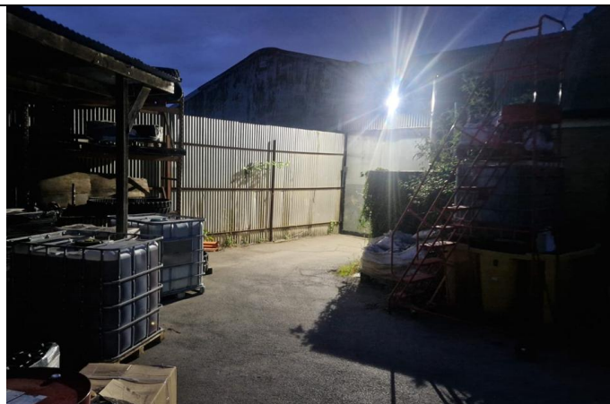
Single LED-chip luminaire, shown in the daytime photo, above the door
