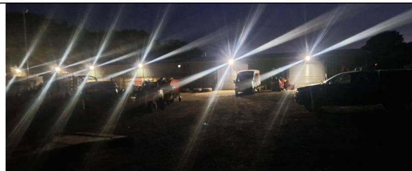
Luminaires on the eastern façade of the building. Glare is evident. Dark spots between the luminaires show the limited optical control associated with the existing luminaires.
