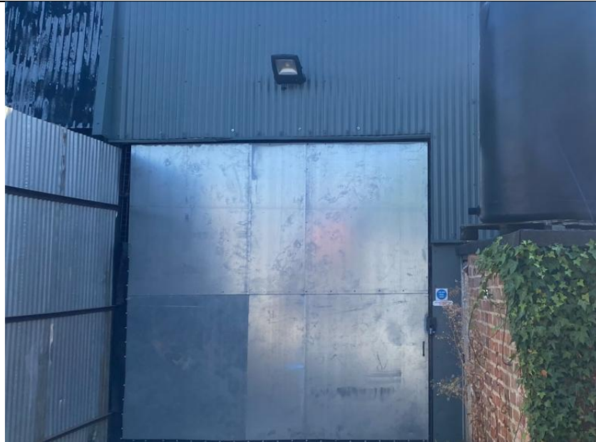
Floodlight above door. Single-chip LED. No branding.
