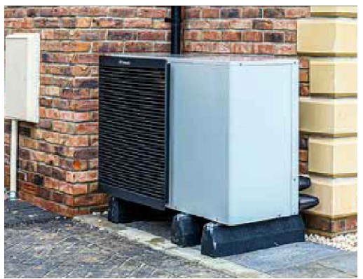
Daikin Altherma 3 M ASHP unit
