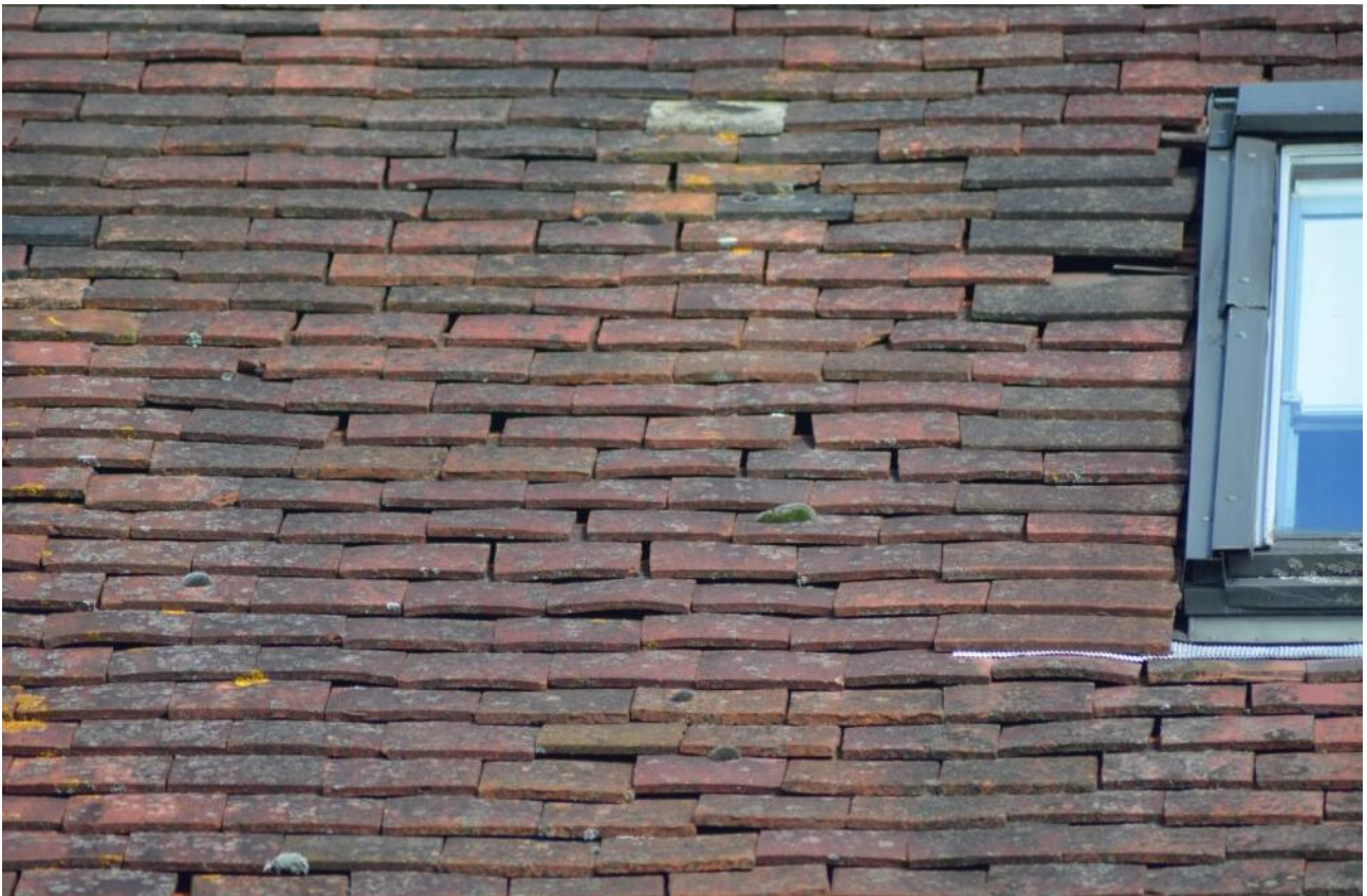
Figure 4: The roof of B1 at Hollyville presents many gaps around roof tiles
