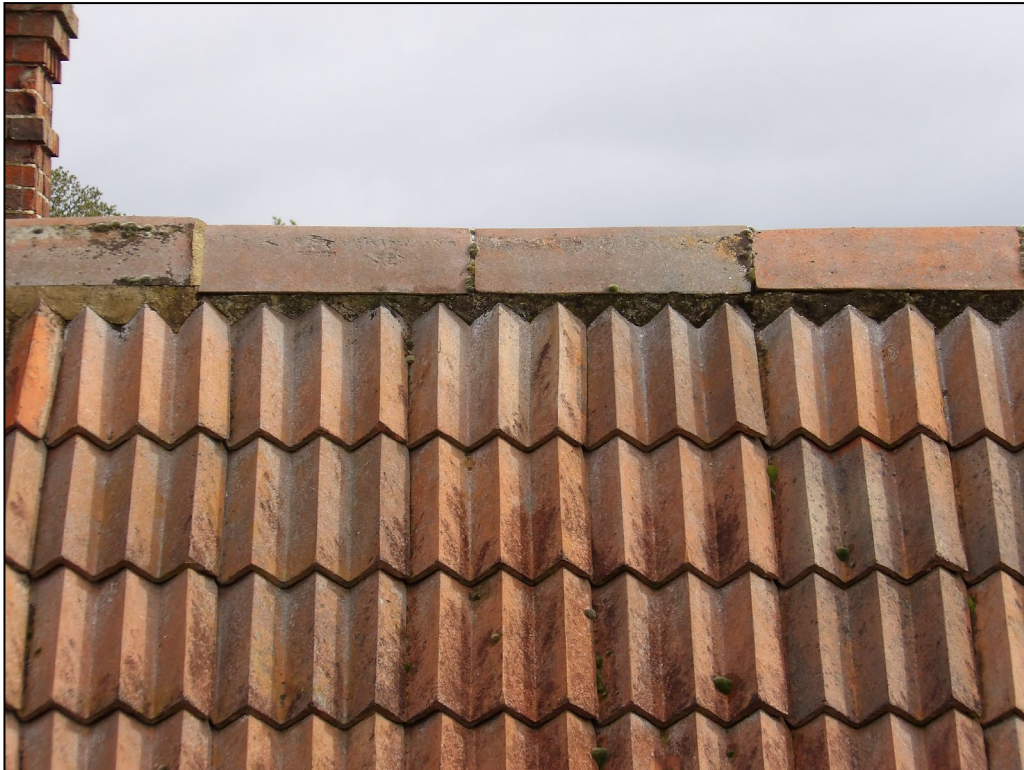
Figure 6. Tightly fitted ridge tiles. 2 Diddenham Cottages, Grazeley. 01.10.24
