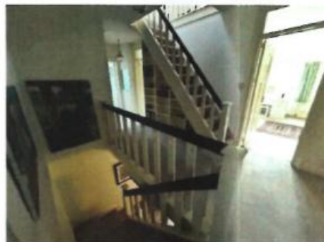
Figure 28: Spindles on balustrades too far apart.
