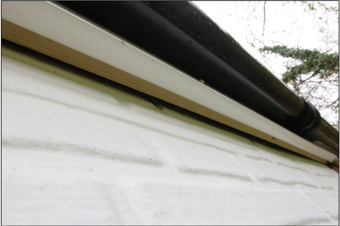
Photo 8: Occasional gap between soffit board and pre-fab wall – no bat evidence noted
