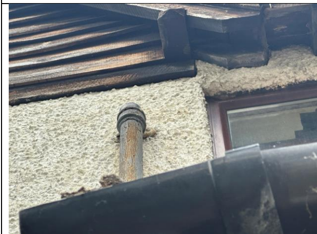
Photo 3 Minor gaps beneath weather boards
