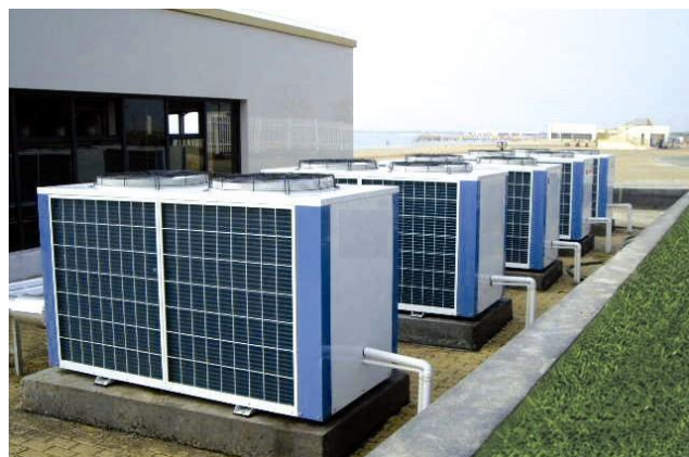
Figure 6: Outdoor units of ASHP.
