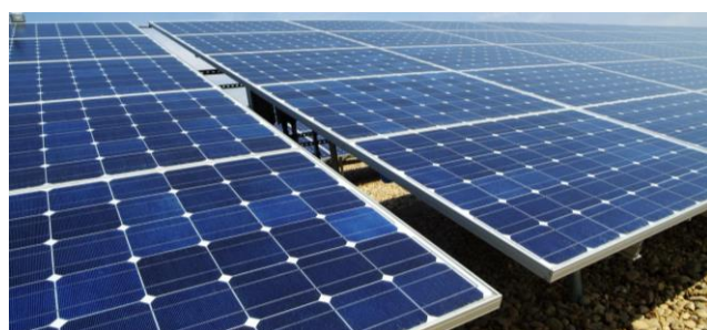
Figure 4: Monocrystalline PV arrays.
