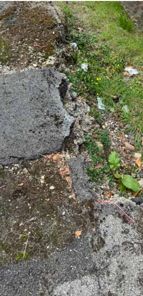
Existing black top + potential trip hazard
