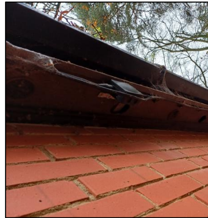
Photo 10 Gap in soffit on maintenance building
