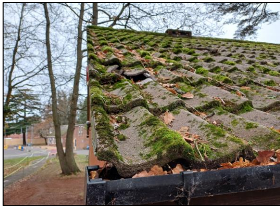
Photo 9 Crack in tile on maintenance building
