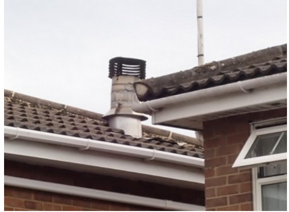
Photograph 6. Lifted lead flashing with open gap beneath (southwestern elevation).
