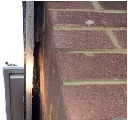
Photograph 8. Cobwebbed gap between fascia and brickwork; open space with no crevice opportunities (rear elevation).
