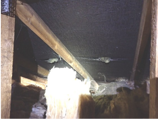
Photograph 13. Overlapping sections of bitumen felt blocked by fibreglass insulation.
