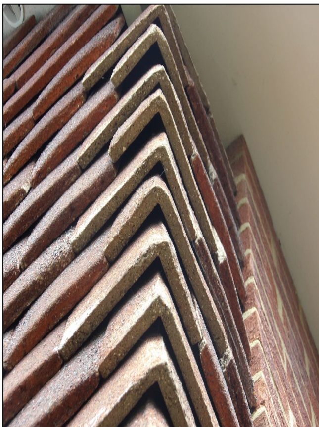
Figure 12. Moved hanging tiles on corner of front elevation. 7 Pine Drive, Finchampstead. 22.04.25
