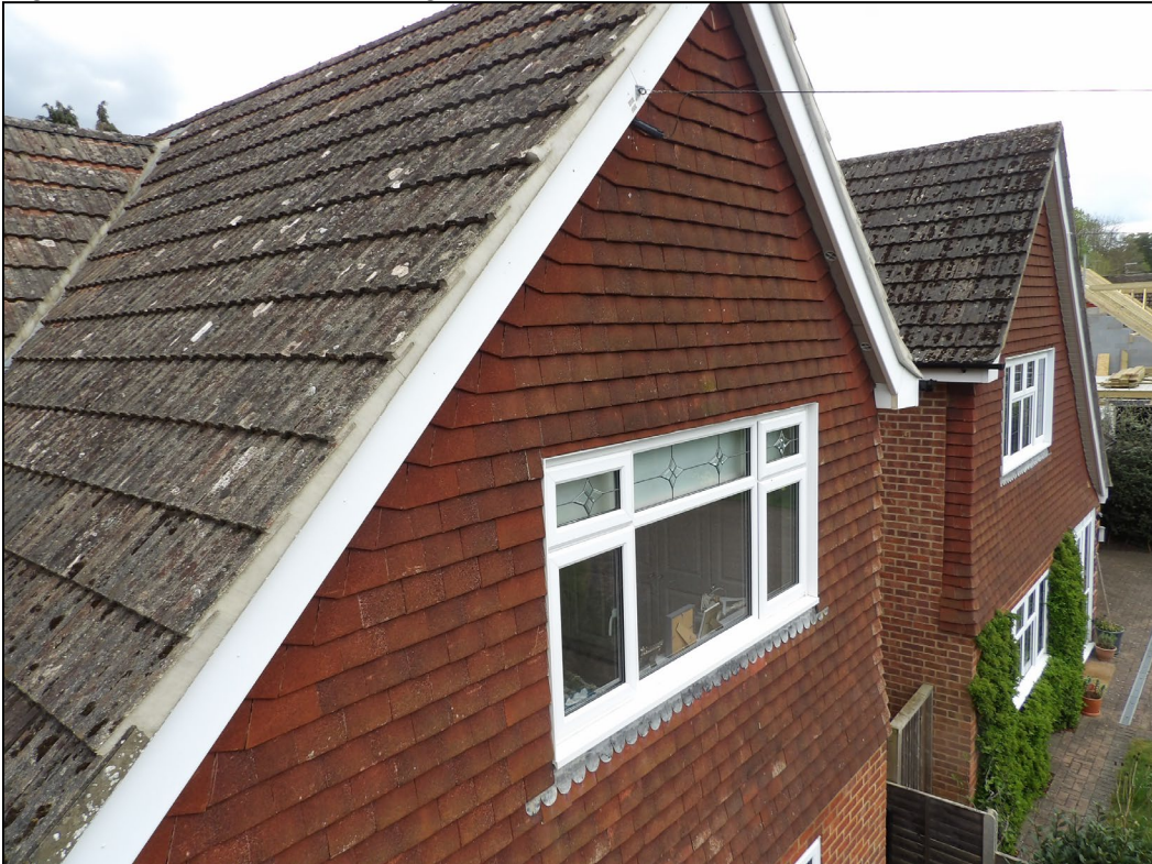
Figure 6. Example sealed verges. 7 Pine Drive, Finchampstead. 22.04.25
