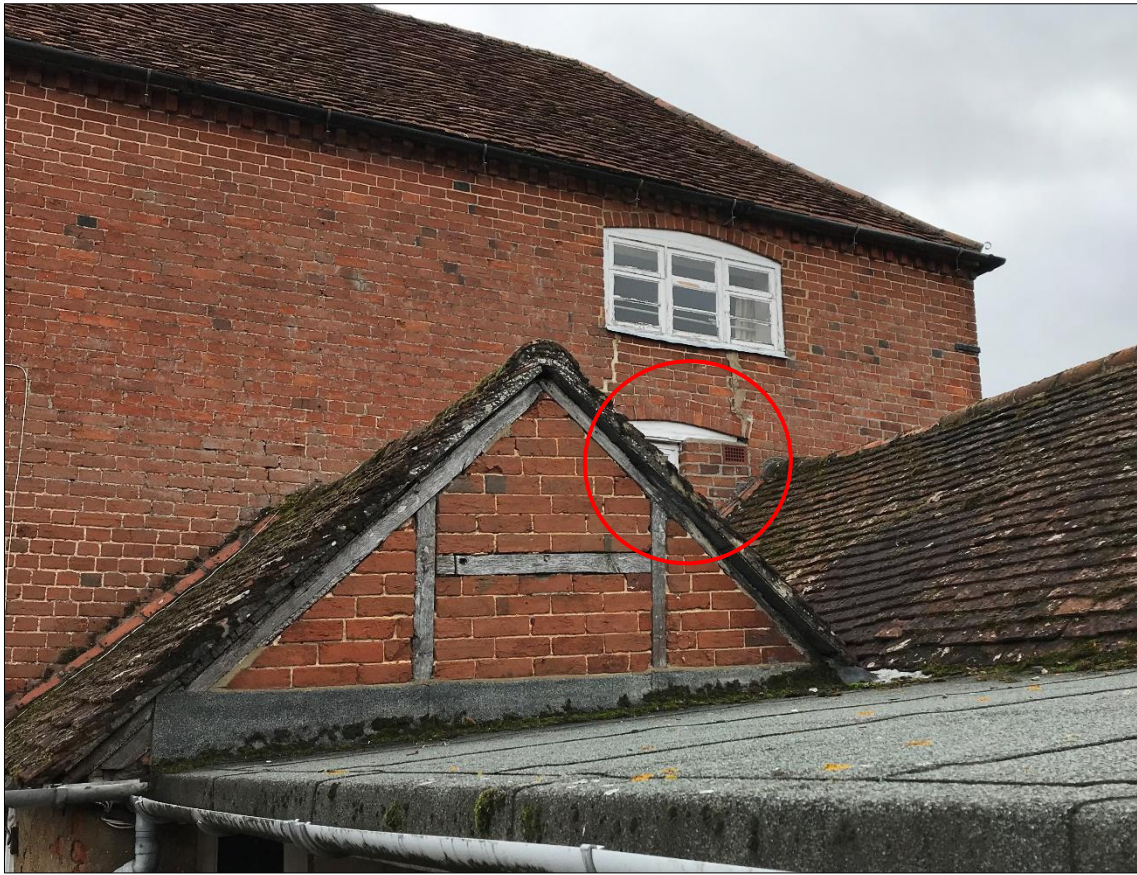
Fig. 13. Farmhouse window partially blocked by the roof of the extension.
