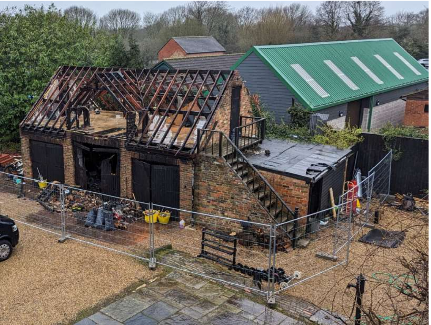
Figure 15. Image showing current fire damage and Shed behind
