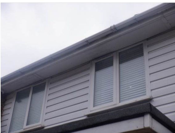
Photograph 7. Interlocking uPVC cladding (front elevation).
