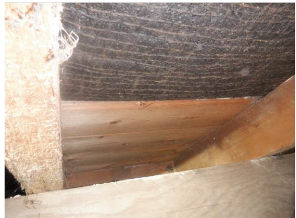
Photograph 14. Tight timber boarding around chimney (roof void).
