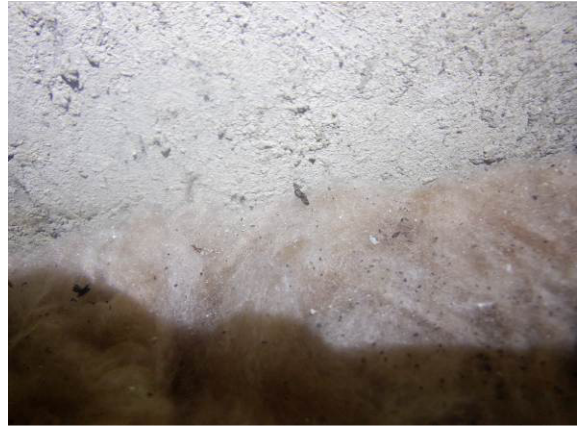
Photograph 16. Small bat dropping at southern gable end (roof void).
