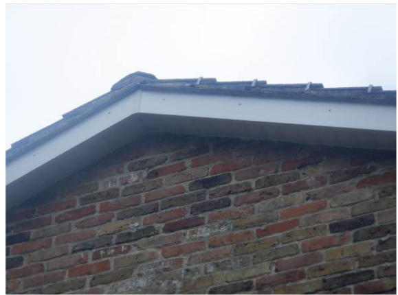
Photograph 6. Gaps in verge mortar (southern elevation).
