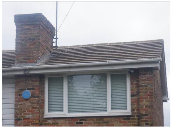
Photograph 4. Mortared ridge tiles and flat lead flashing (front elevation).
