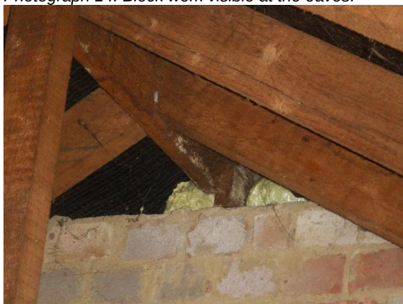
Photograph 16. Expanding foam at the apex of the western internal gable end wall.
