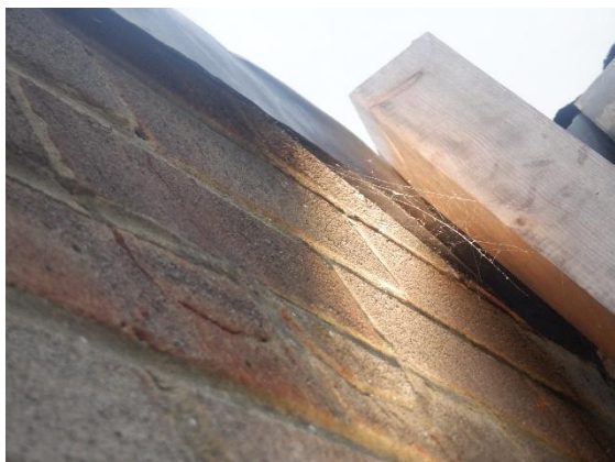
Photograph 11, Slight gap behind plastic on the roof of the garage.
