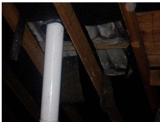
Photograph 13. Large tear in the roofing felt
