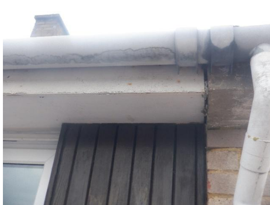
Photograph 8. Timber cladding tight to the front of the bungalow.
