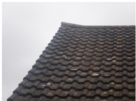
Photograph 5. Ridge tile slightly lifted with mortar visible behind.
