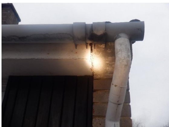
Photograph 7. Superficial gap in soffit to the front of the bungalow.
