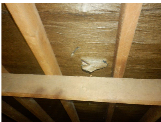
Photograph 9. Section of roof with paper backed felt with occasional tears.
