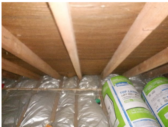
Photograph 11. Foil covered fibreglass insulation at roof margins.
