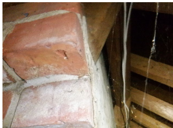
Photograph 12. The chimney tight to the roof and cobwebbed.
