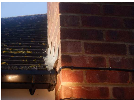
Photograph 7. Tightly fitted lead on side of southernmost chimney with open gap of negligible extent by gutter.
