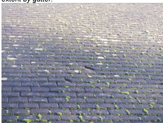
Photograph 9. Broken tiles on the western elevation not leading to gaps suitable for bats.
