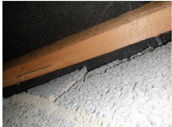
Photograph 14. Blockwork tight to roofline and felt.
