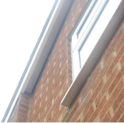
Photograph 5. Gap between soffit and brickwork on the western front gable.
