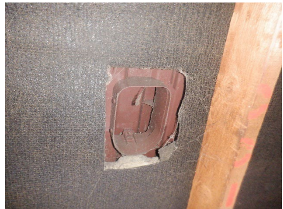
Photograph 10. Gap in bituminous roofing felt around plastic vent tile.
