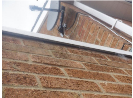
Photograph 8. Barge board tight to brickwork on bay window.
