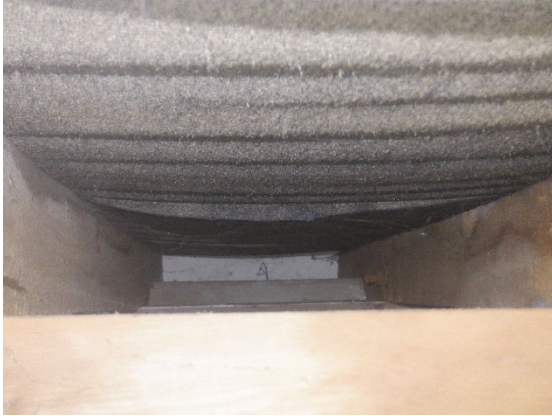
Photograph 11. Eaves open to the soffit on the eastern side.
