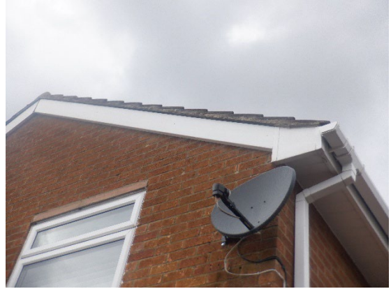
Photograph 6. Barge board tight to brickwork on the eastern front gable.
