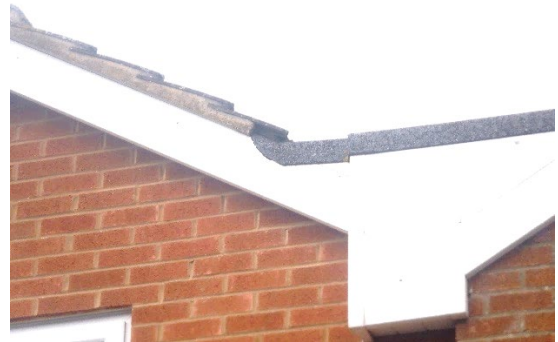
Photograph 4. Section of mortar missing from bottom of verge to the front of the house.
