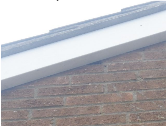
Photograph 7. Section of missing brickwork on the rear gable creating a gap under the barge board.
