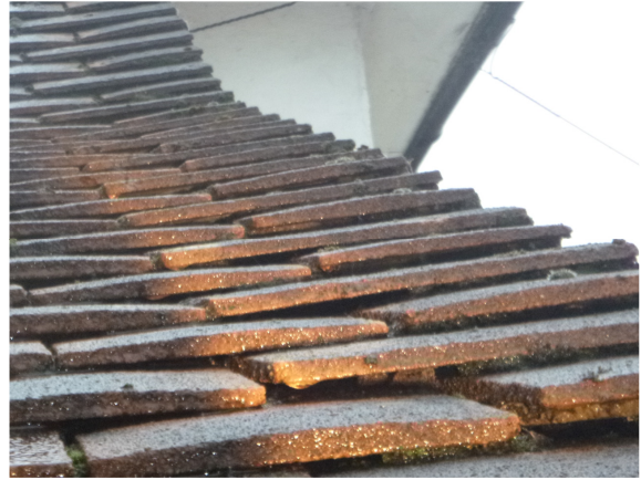
Photograph 2. Lifted roof tiles across the front catslide roof (front elevation).
