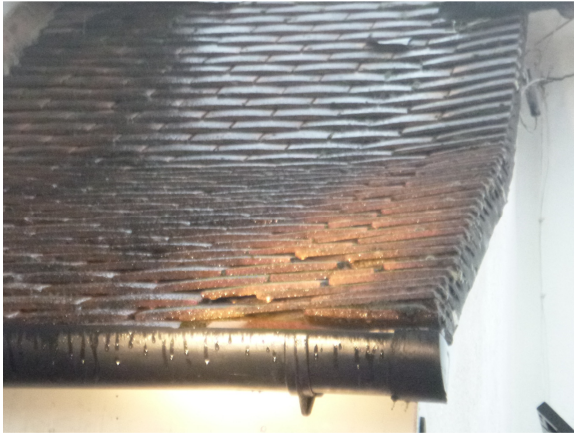
Photograph 1. Lifted roof tiles across the front catslide roof (front elevation).
