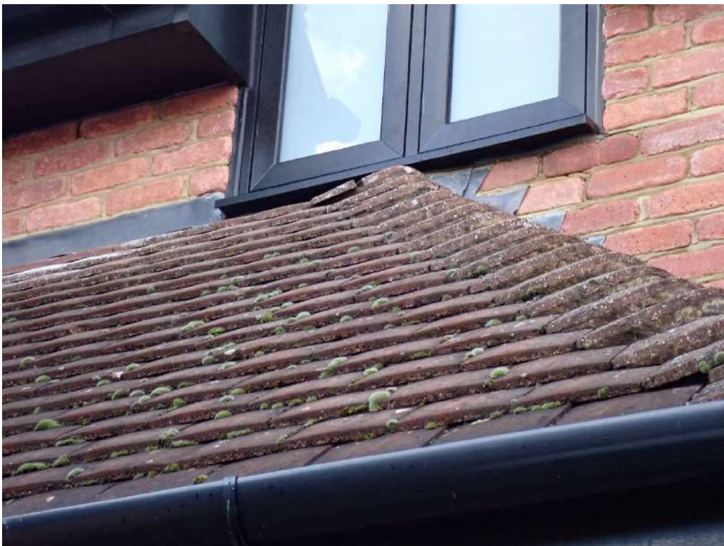
Photograph 4 – Small sections of missing mortar under hip tiles on the eastern aspect.
