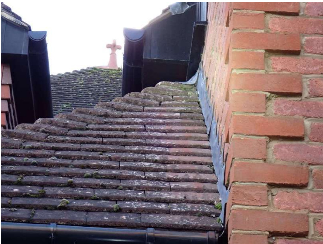
Photograph 10 – Raised lead flashing between the porch and eastern aspect window.
