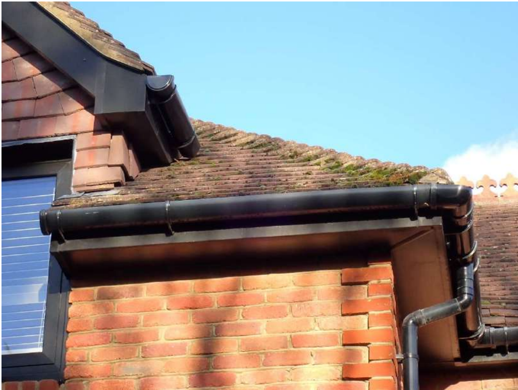
Photograph 7 – Example of raised hanging tiles associated with one of the dormers.
