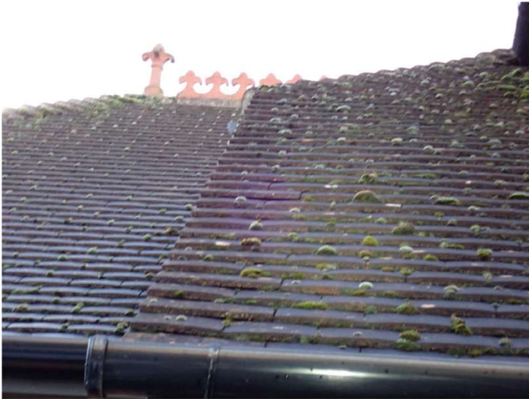
Photograph 3 – Raised roof tiles on the eastern aspect.
