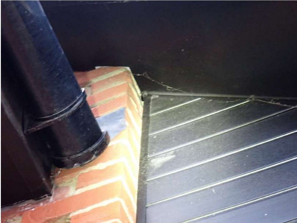
Photograph 11 – Gap beside plastic weather boarding above front door.
