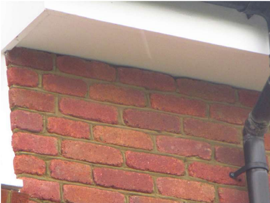
Photograph 20 – Photograph from the original scoping survey conducted on 05.01.21, showing slight gaps between the wall plate and the boxed soffits.
