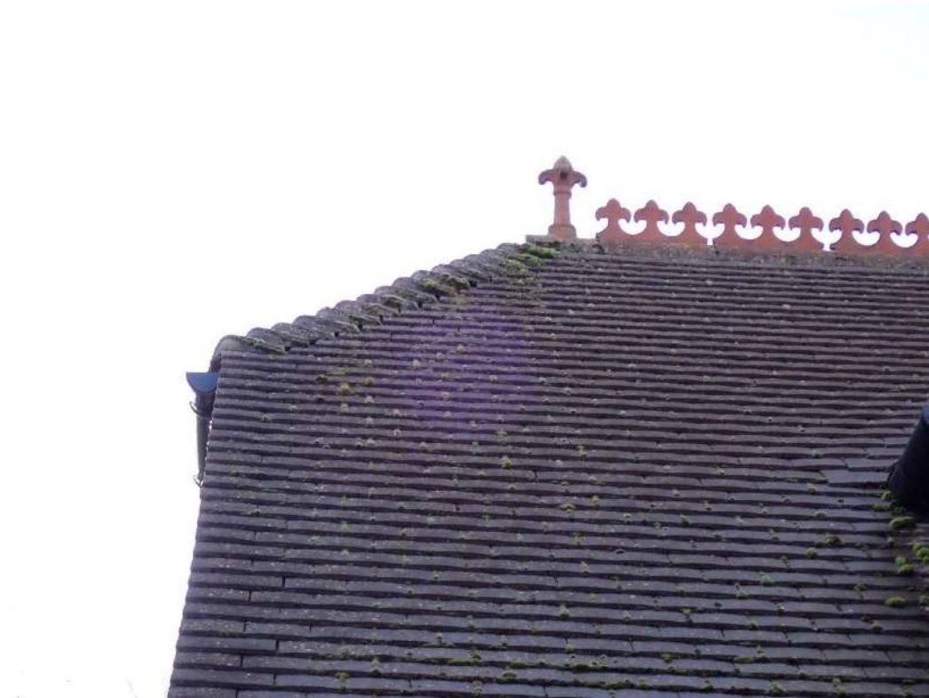
Photograph 5 – Gaps along the hip tiles at the southeastern aspect of the building.
