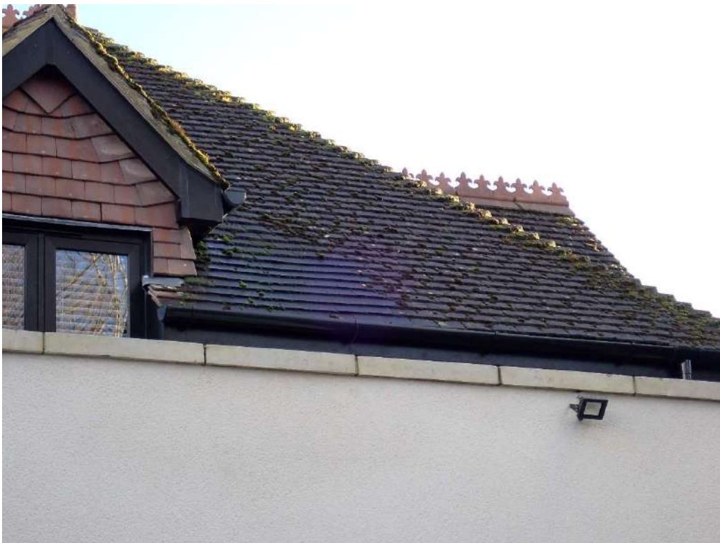
Photograph 8 – Example of raised lead flashing on the dormer at the northern aspect of the building.
