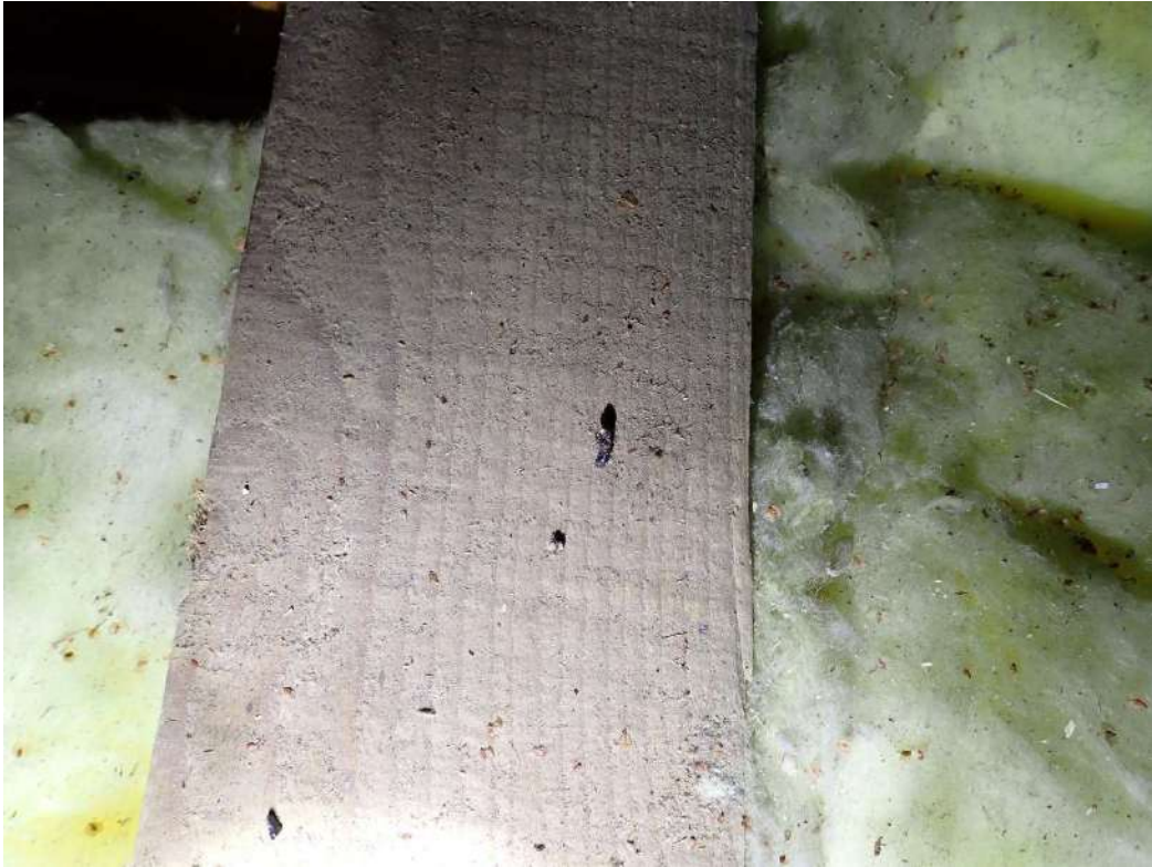
Photograph 19 – Single bat droppings identified near access hatch.
