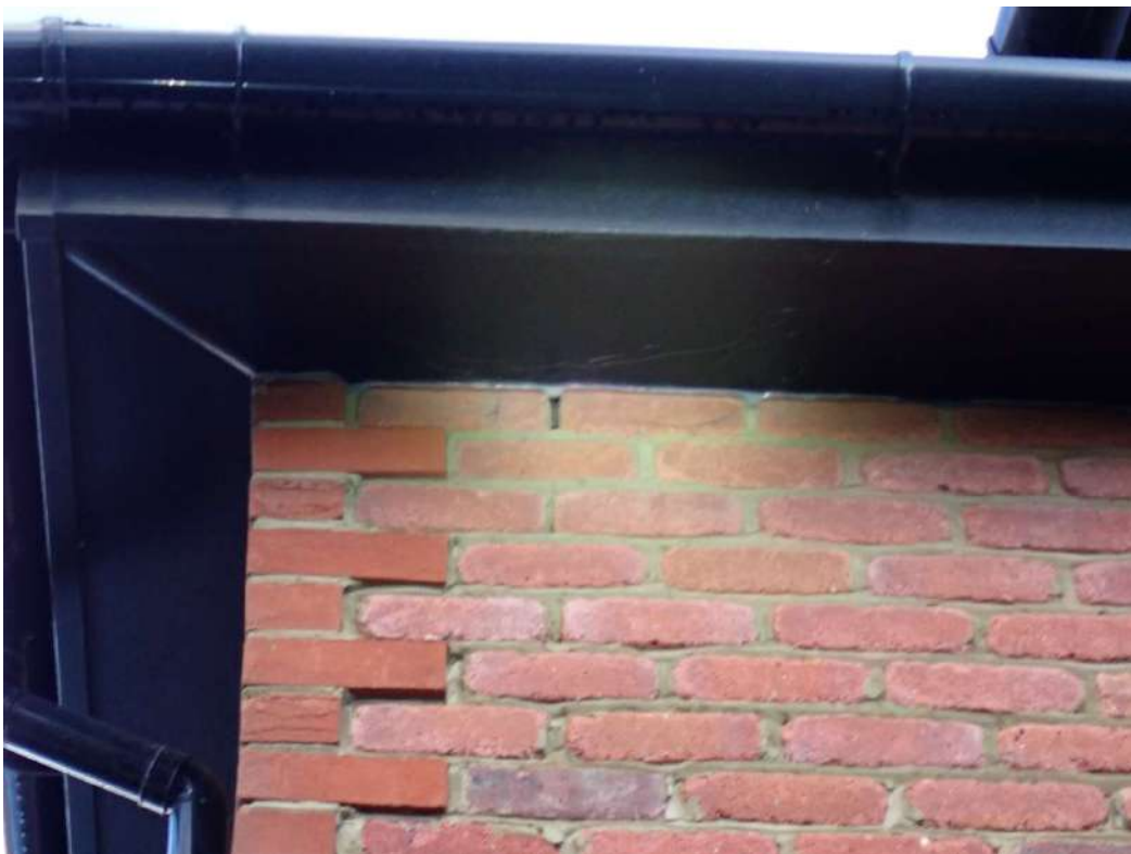
Photograph 12 – Mortar crevice within brickwork at wall plate on the western aspect of the building.
