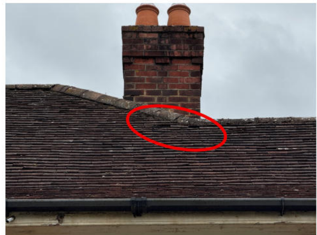
Gaps under roof tiles on northern aspect.
