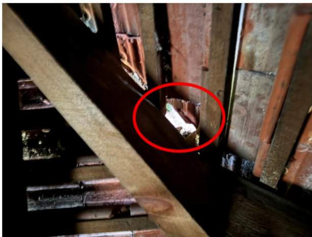
Gap at roof junction next to eastern chimney breast.
