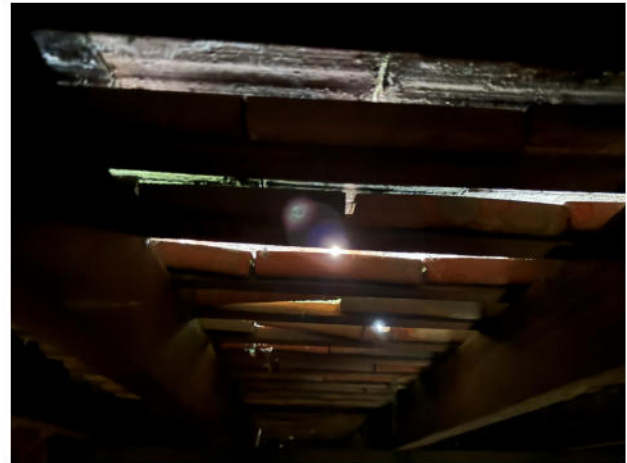
Gaps between roof tiles on eastern aspect.
