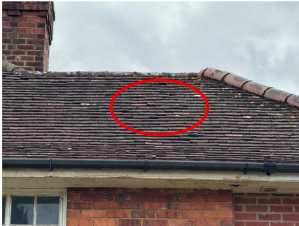
Gaps under roof tiles on northern aspect.
