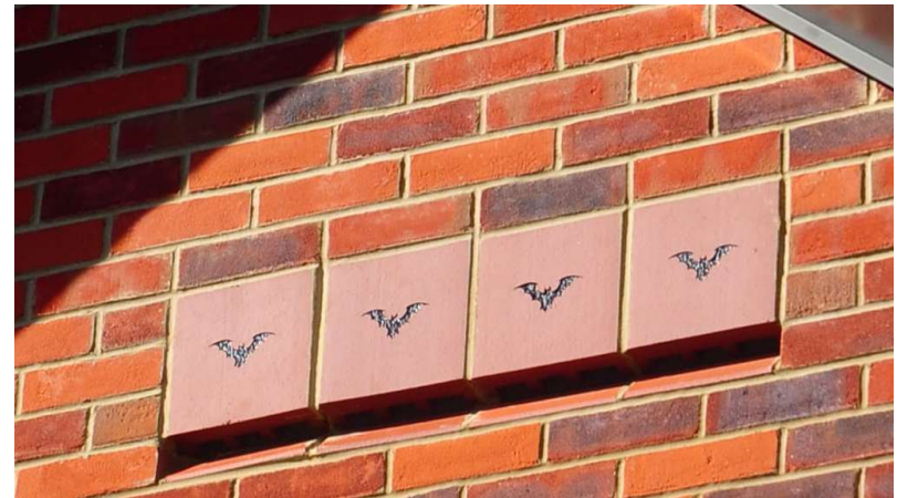
(ii) Bat Bricks Built into Property
