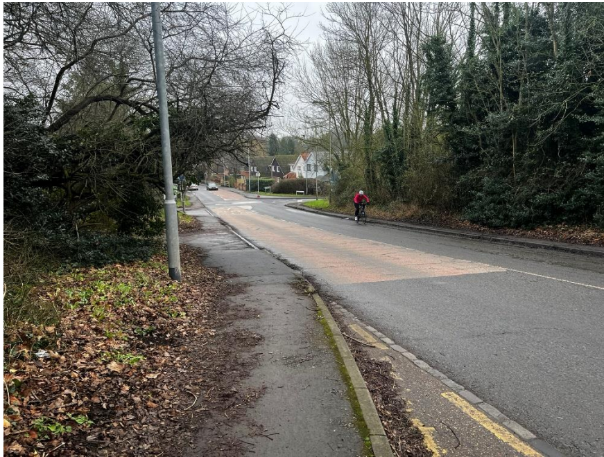
Photograph 8: Condition of Barkham Road
