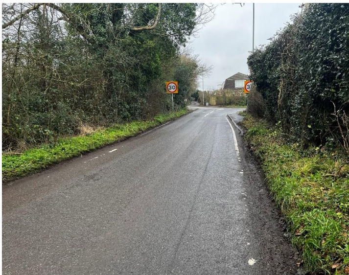
Photograph 6: Condition of Edneys Hill
