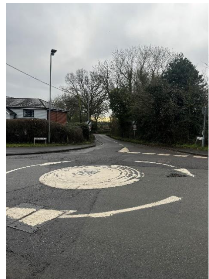
Photograph 7: Condition of Edneys Hill/B3349 Barkham Road mini roundabout
