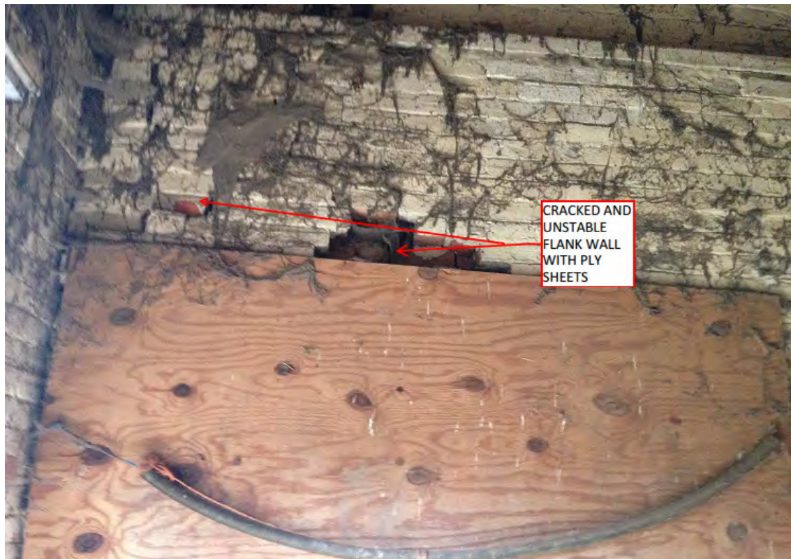
DEFECTS OBSERVED IN BUILDING 'D' & 'E'
