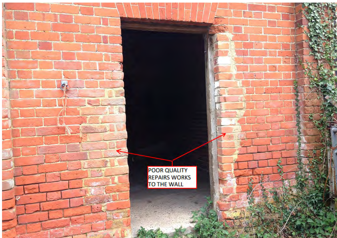
DEFECTS OBSERVED IN BUILDING 'D' & 'E'
