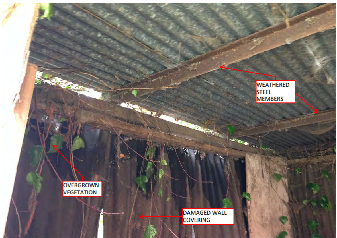
DEFECTS OBSERVED IN BUILDING 'B'
