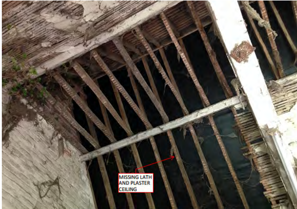
DEFECTS OBSERVED IN BUILDING 'D' & 'E'
