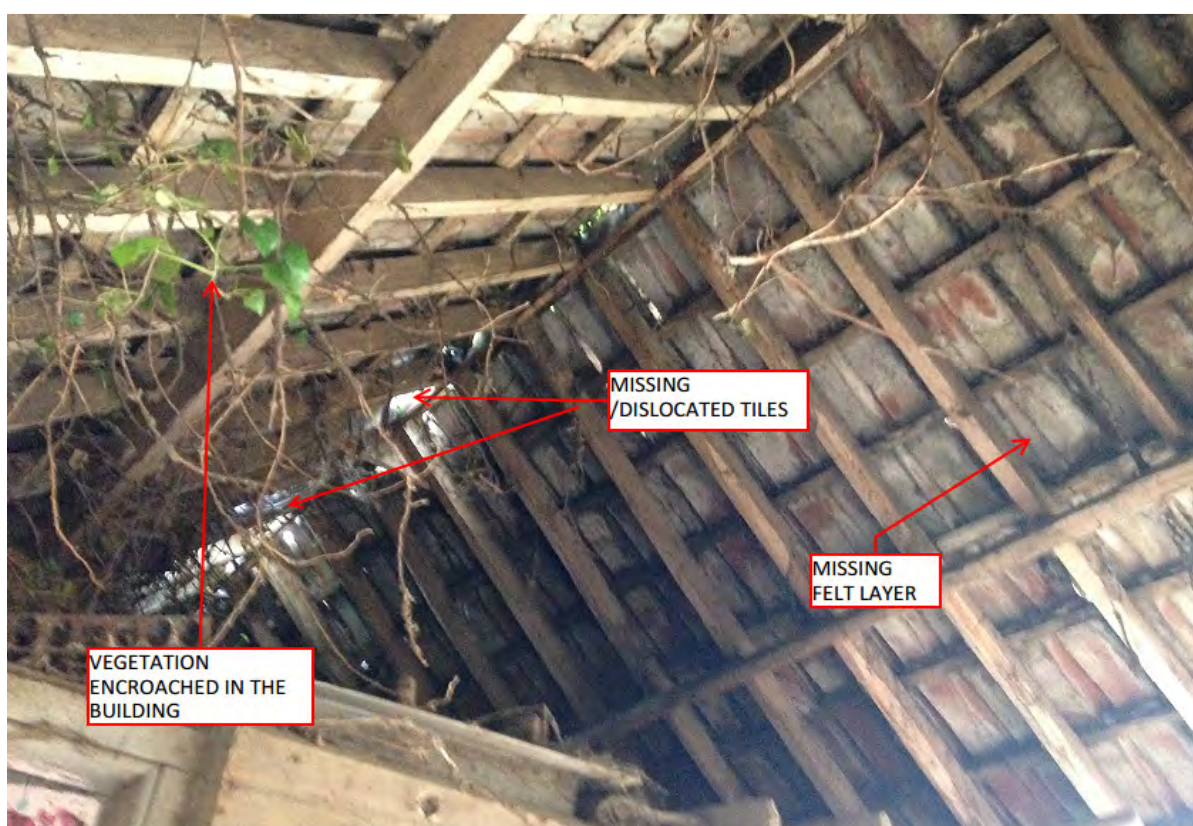
DEFECTS OBSERVED IN BUILDING 'C'
