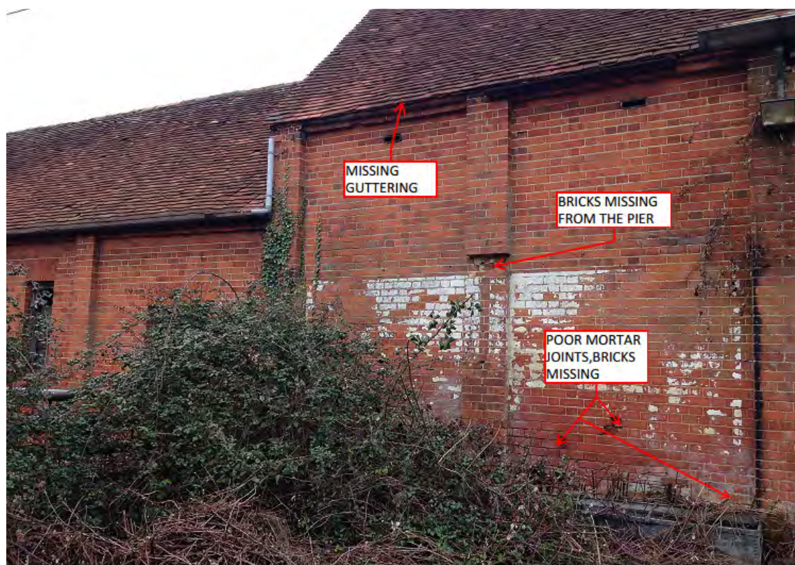
DEFECTS OBSERVED IN BUILDING 'K'
