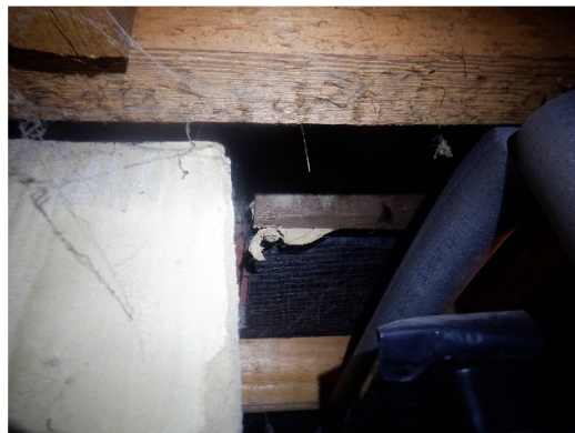
Photograph 11. Large tear in the roofing felt..
