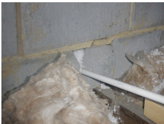
Photograph 16. Shredded fibreglass visible in gable end.
