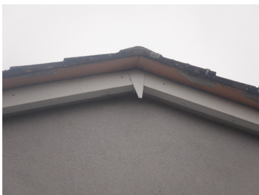
Photograph 5. Fascia tight to the rendered walls at the gable end to the front of the house.
