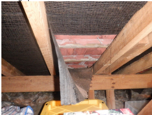
Photograph 12. Large tear in the roofing felt.
