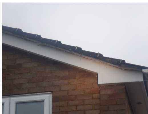
Photograph 6. Superficial gap in the verge mortar on the rear gable end.
