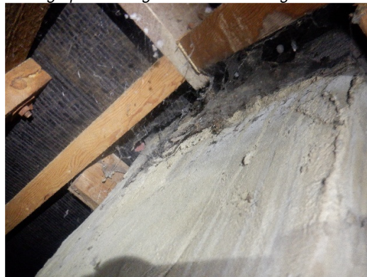
Photograph 13. Gap in felt at side of the chimney.
