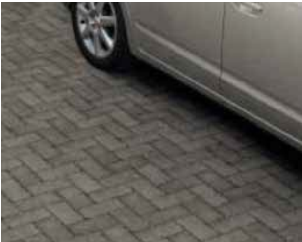
Pakring Bays - Permeable blocks
