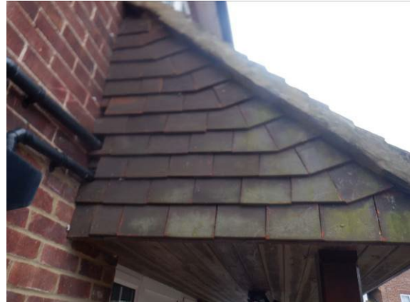
Photograph 9. Lifted hanging tiles (front elevation).
