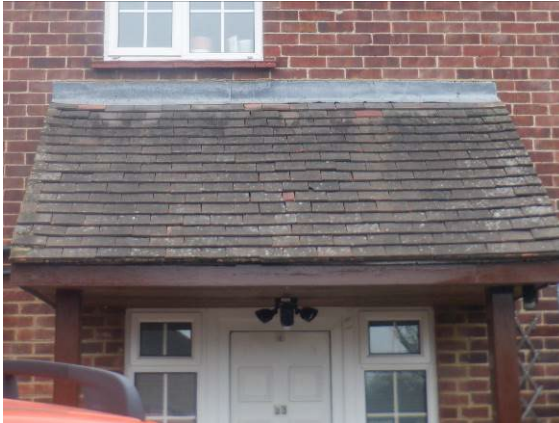
Photograph 8. Occasionally uneven roof tiles (front elevation).
