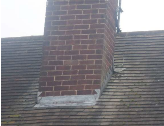
Photograph 6. Lead flashing slightly lifted around chimney (rear elevation).
