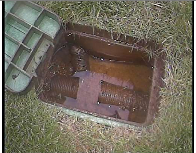
Access problems: RE2 FULL OF WATER
