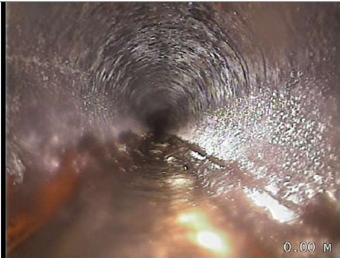
Start node type, manhole, reference FWMH2
