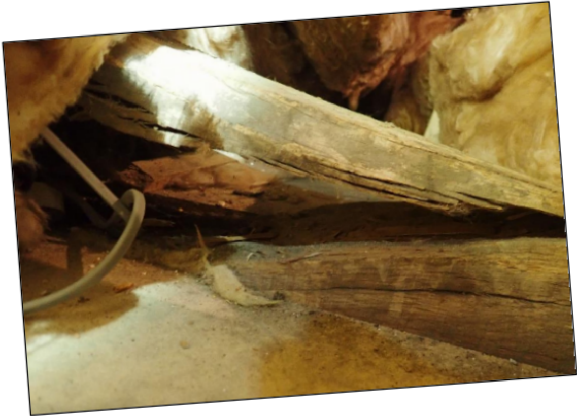
Figure 43. View of the fracture in the 1 st -floor ceiling beam
