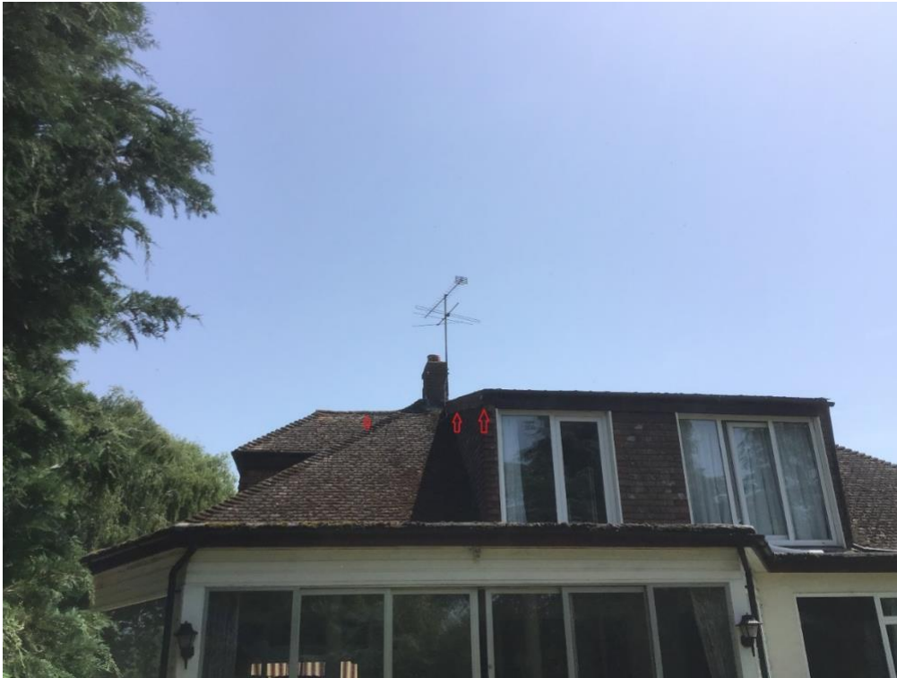
Figure 3. Northern elevation looking east. Red arrows indicate potential access points into under-tile spaces.
