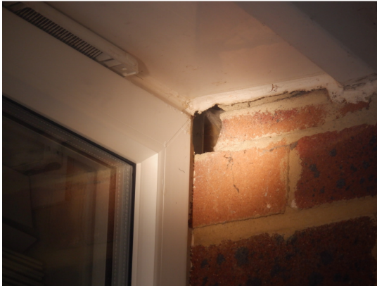
Photograph 10. Gap in the corner of the soffit box filled with fibreglass.
