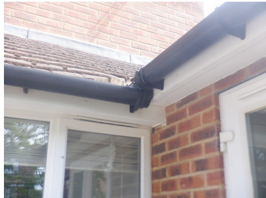
Photograph 9. Gap in the corner of the soffit box.
