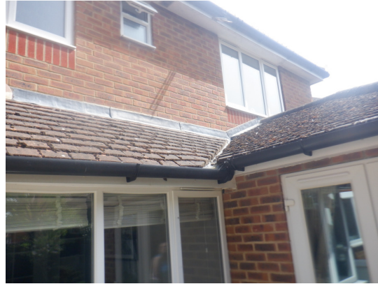
Photograph 7. Tight led flashing between hipped roof and brick work of rear extension.
