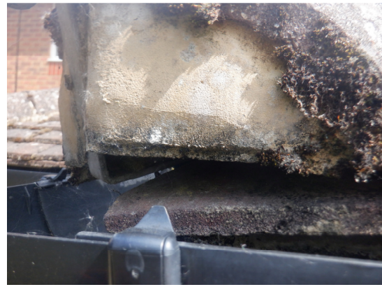
Photograph 5. Small gaps at between hip mortar and plain roof tile.
