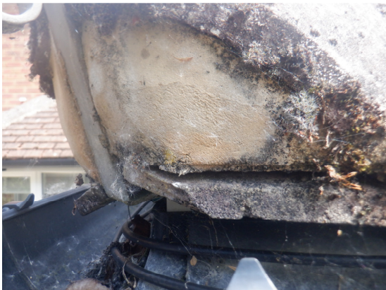
Photograph 4. Small gaps at eaves between hip mortar and roof tile.
