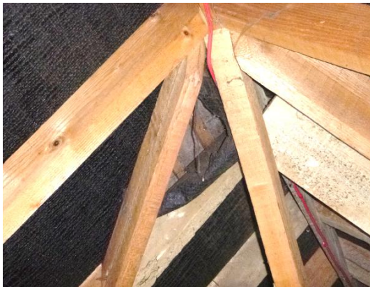
15. Small tear in roofing felt.
