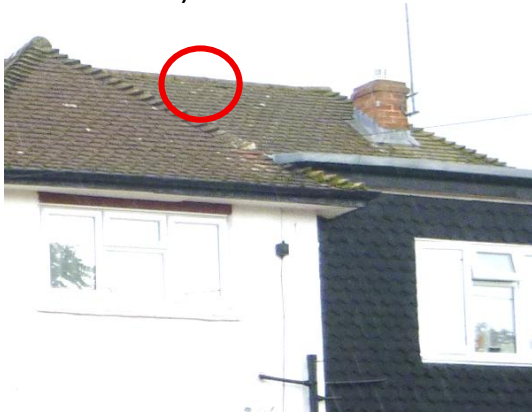
5. Missing roof tile beneath ridge (front elevation).
