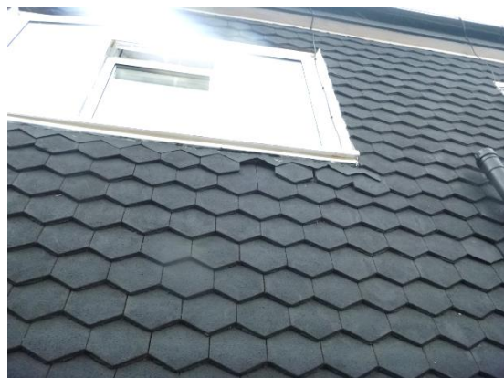
8. Missing hanging tile (front elevation).
