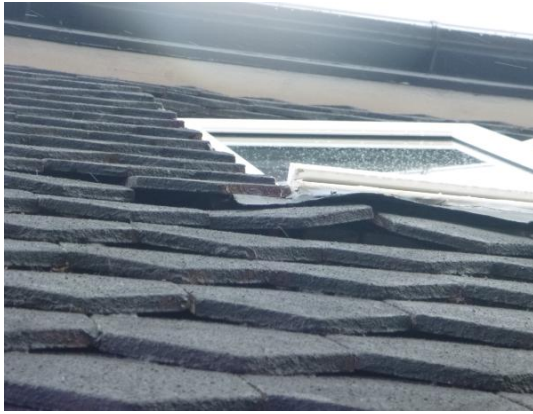
9. Slight gaps behind hanging tiles (front elevation).
