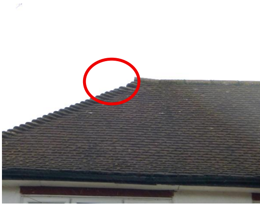
3. Missing mortar beneath hip tile (front elevation).
