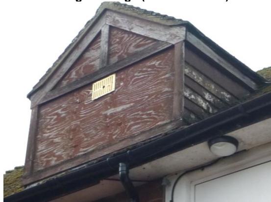
6. Gaps to rear of timber dormer (rear elevation).
