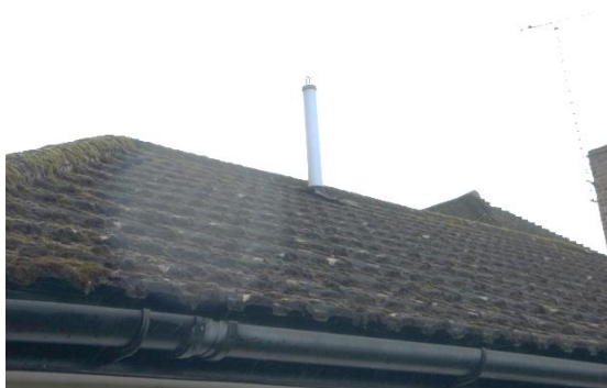
12. Gap beneath flashing around flue (western elevation).
