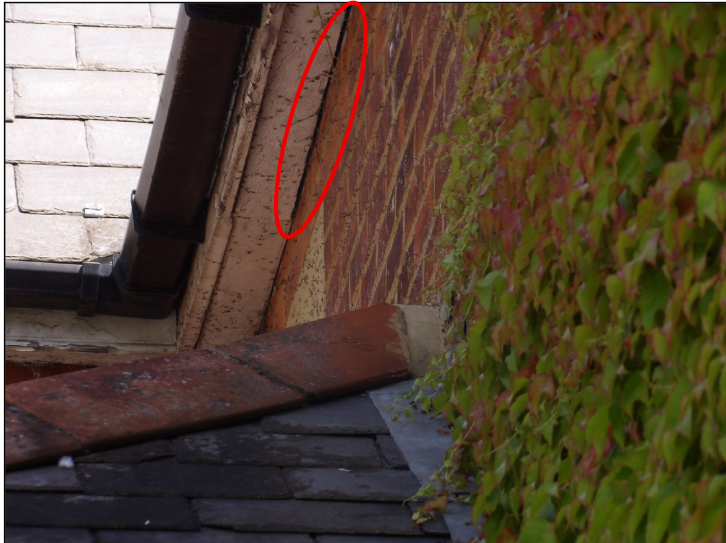
Figure 8. Example gap in soffits/wall plate. Lea Heath House, Hurst. 23.06.26
