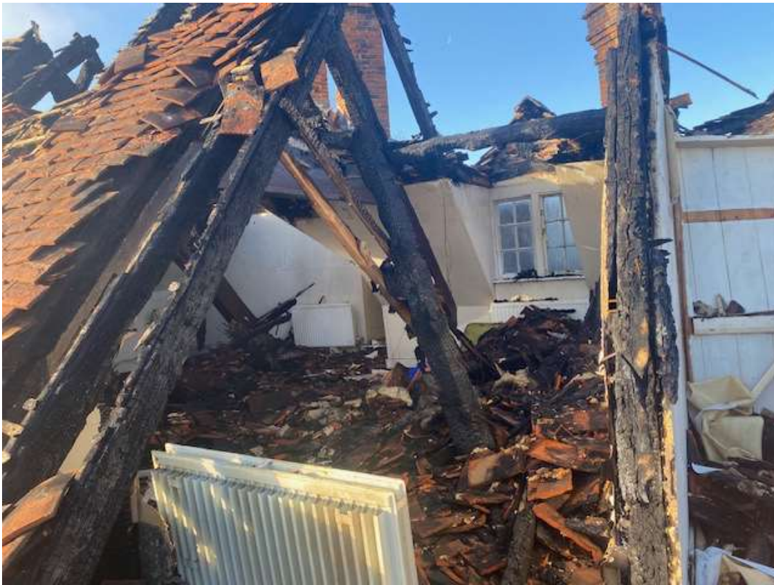
Photograph 4, 5 & 6—fire damaged roof structure
