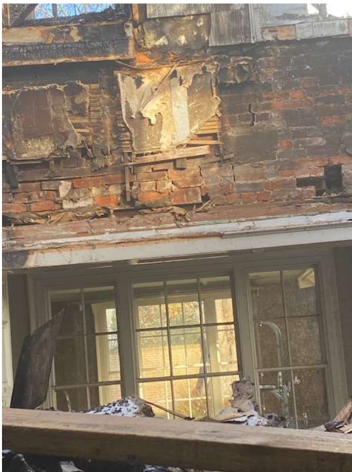
Photograph 3 – Possible historic crack in wall over alcove
