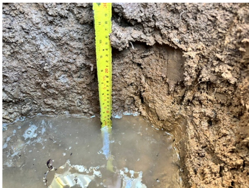
Photo 1 – Excavation with Ground Water
