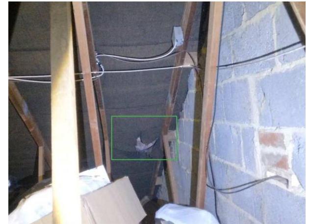
B1 - Internal void LV1 hole in lining
